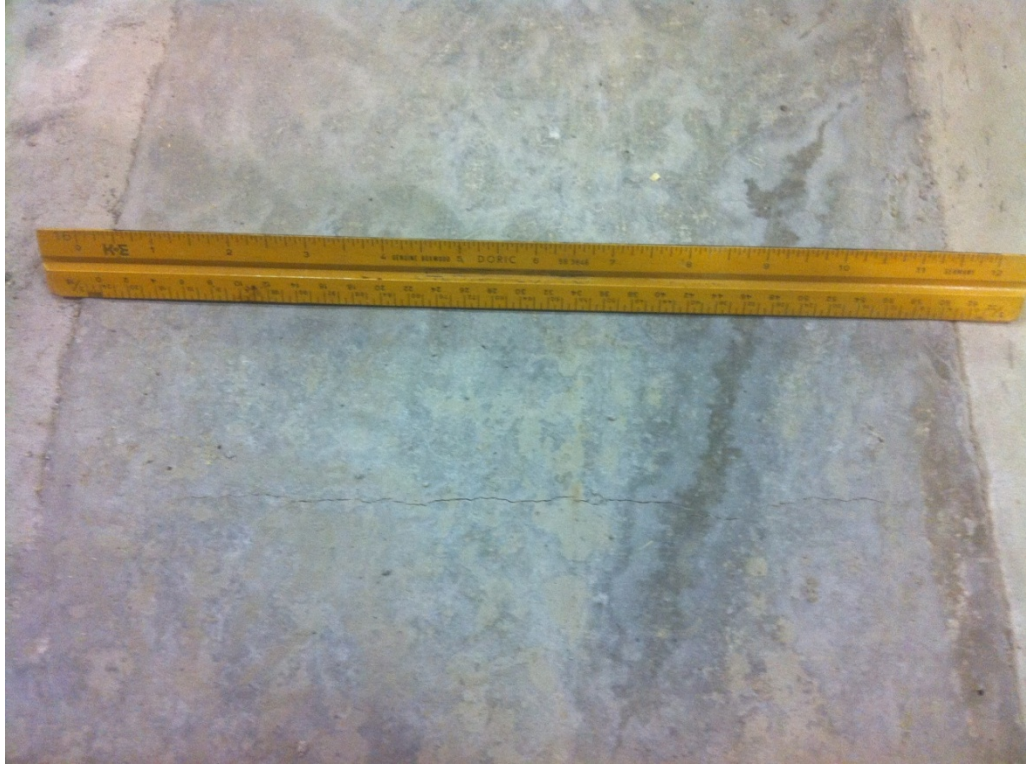
Figure 4-37: Shrinkage Cracking across Staged Construction Joint
