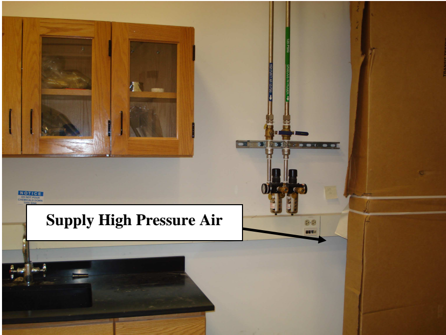
Figure 2.10 High pressure air line
