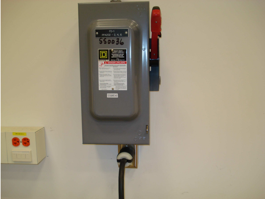
Figure 2.12 Braiding machine main power quick disconnect
