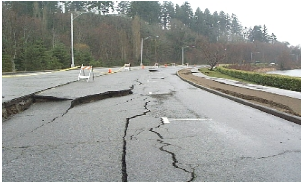
Figure 2.12: Ground failure showing lateral spread after 2001 Nisqually earthquake Olympia, Washington ( http://peer.berkeley.edu/nisqually/geotech/liquefaction/lateralspread/ ).
