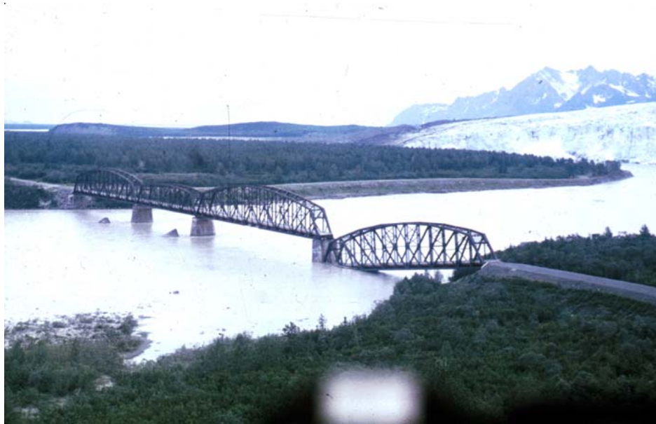
Figure 2.3: Span collapse of the “Million Dollar” bridge due to lateral spreading after the 1964 “Good Friday” earthquake
