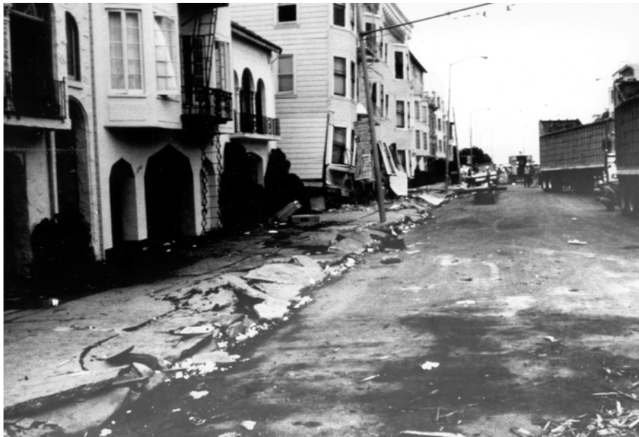
Figure 2.5: Liquefaction induced damage in the Marina District, San Francisco after the Loma Prieta earthquake ( http://libraryphoto.er.usgs.gov/earth1.htm ).
