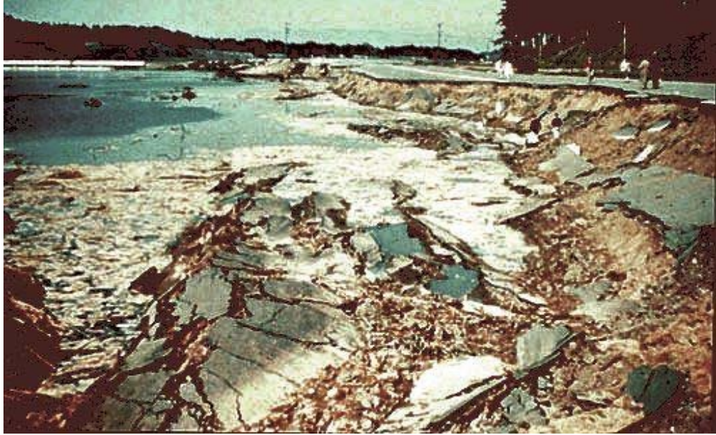
Figure 2.9: Flow failure at Lake Merced, CA 1957
