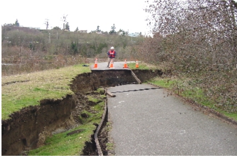
Figure 2.13: Lateral spread of embankment after 2001 Nisqually earthquake Olympia, Washington. The drop seen varies between 3 to 4 feet ( http://peer.berkeley.edu/nisqually/geotech/liqufaction/lateralspread/ ).
