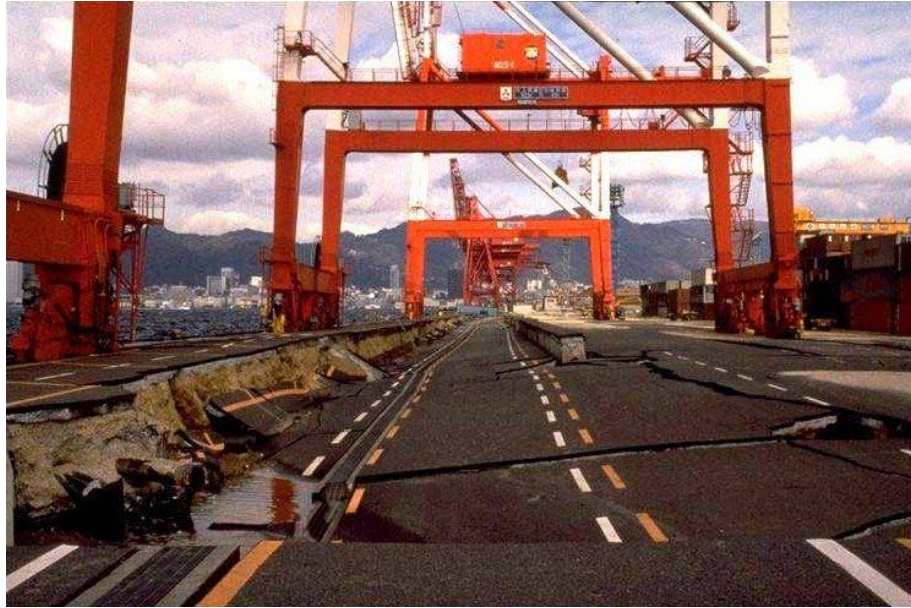
Figure 2.7: Damage at Kobe port due to liquefaction of the underlying fill after the 1995 Hyogo-Ken Nanbu earthquake ( http://www.ce.washington.edu/~liquefaction/ ).
