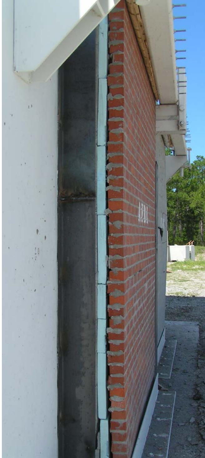
Fig. 3.37. Side view of Wall 2 after Detonation 1
