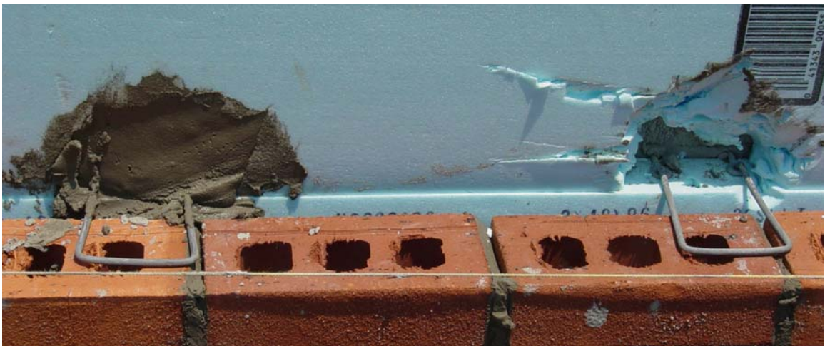
Fig. 5.29. Actual constructed condition of wall ties
