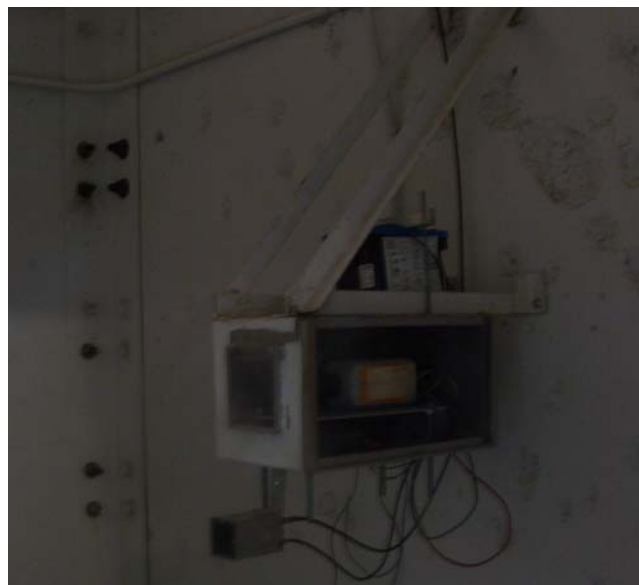
Fig. 3.30. Mounting of an interior camera
