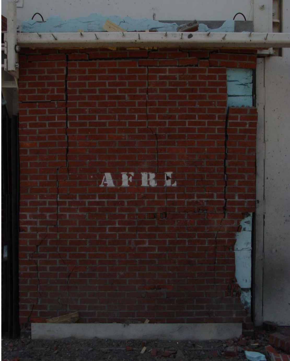
Fig. 3.50. Exterior view of Wall 3 after Detonation 3
