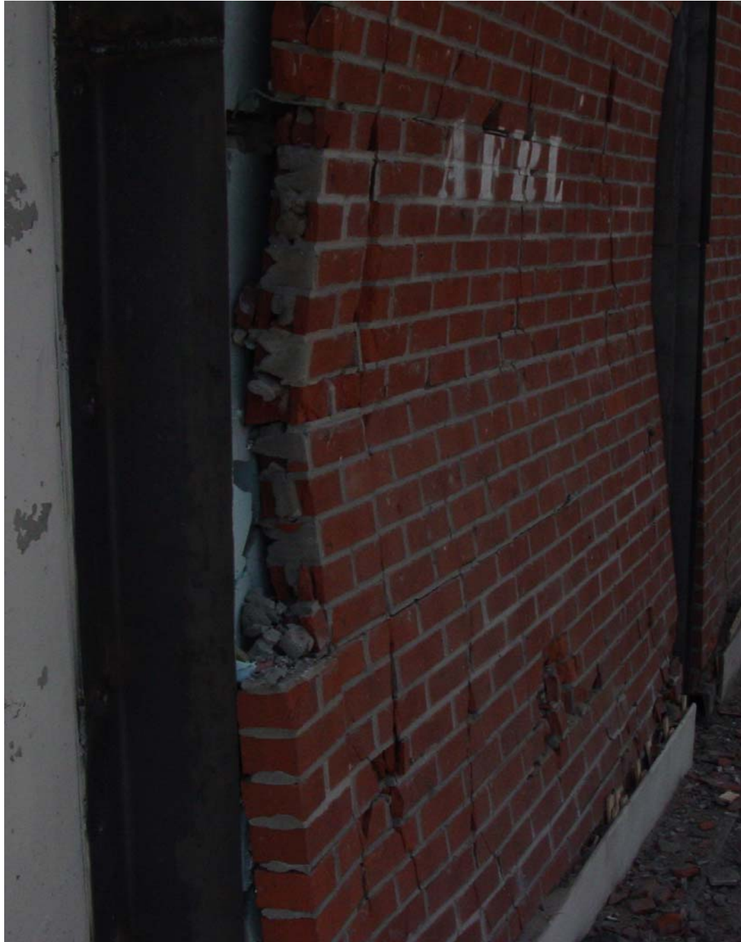
Fig. 3.51. Side view of Wall 2 after Detonation 3
