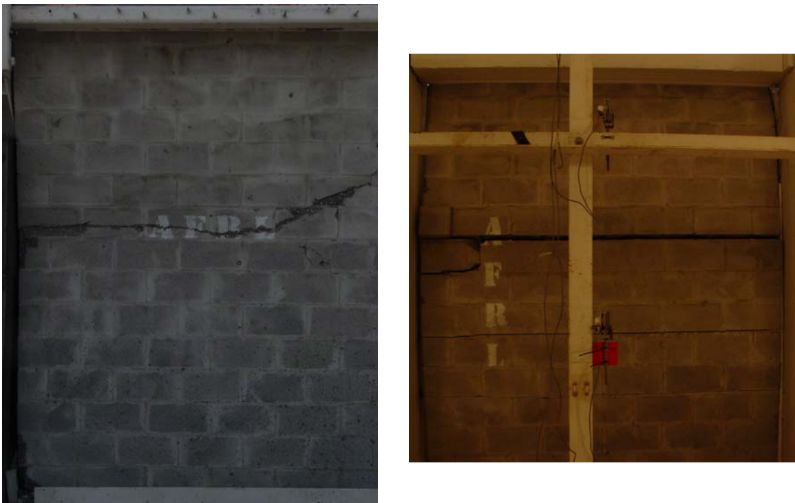
Fig. 3.45. Exterior and interior views of Wall 1 after Detonation 2
