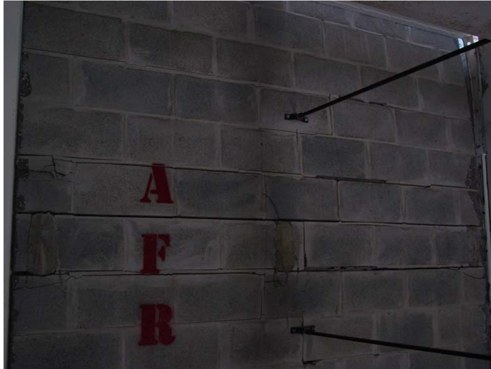
Fig. 3.54. Interior view of Wall 3 after Detonation 3
