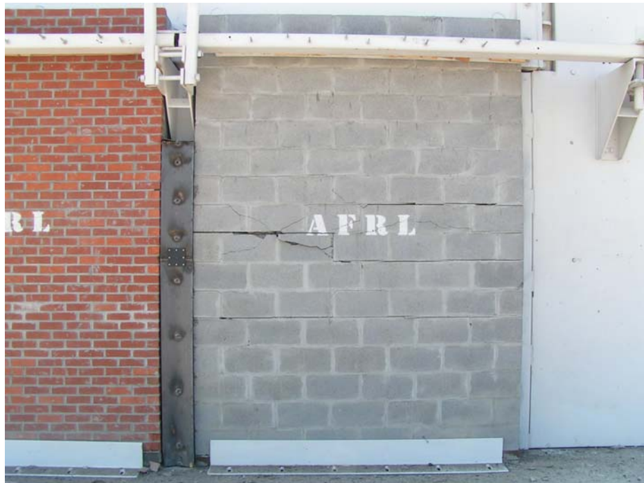
Fig. 3.35. Exterior view of Wall 1 after Detonation 1
