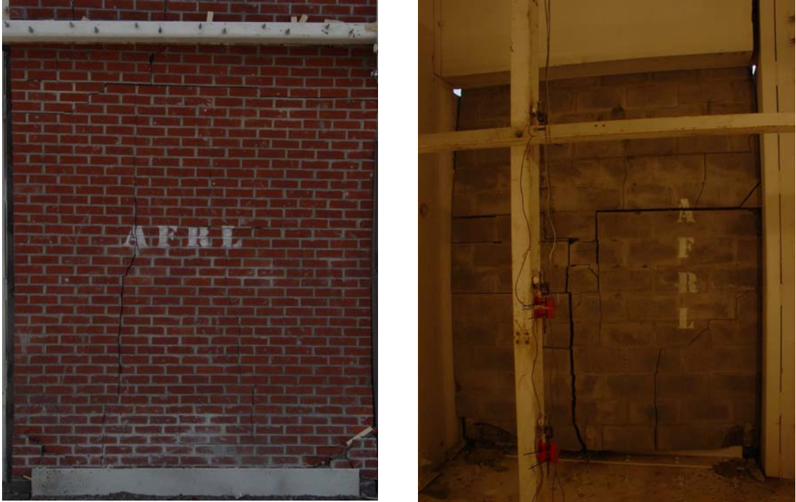
Fig. 3.43. Exterior and interior views of Wall 3 after Detonation 2
