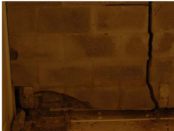
Fig. 3.44. Bottom support failure of Wall 3 in Detonation 2
