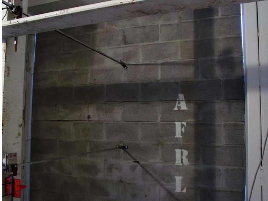
Fig. 3.38. Interior view of Wall 2 after Detonation 1
