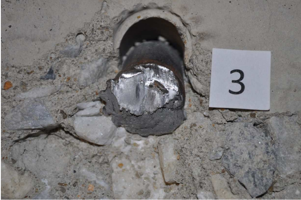
Figure 4-10 Failure Surface for S-0.875-22-C (3)
