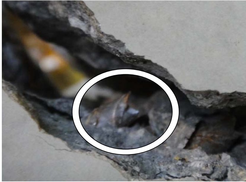
Figure 5-21 Ruptured Tension Steel
