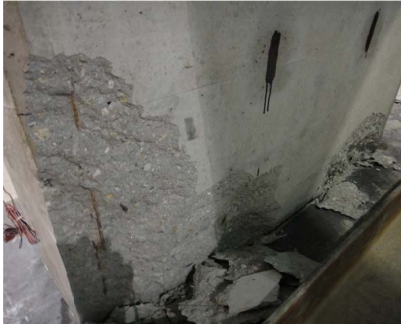
Figure 5-12 Initial Spalling on Bridge Leg
