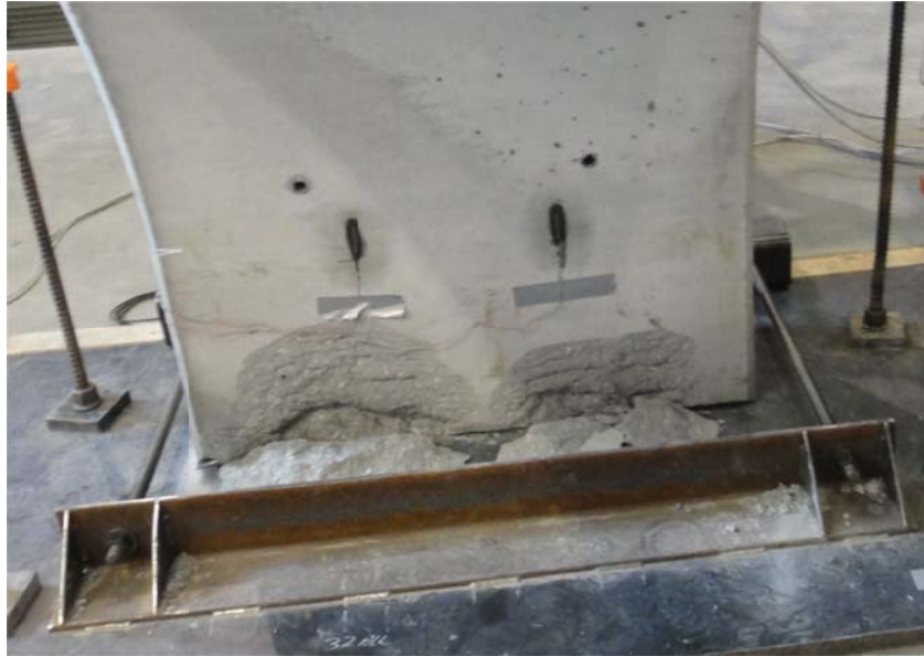
Figure 5-13 Spalling at 96 kips Total Load
