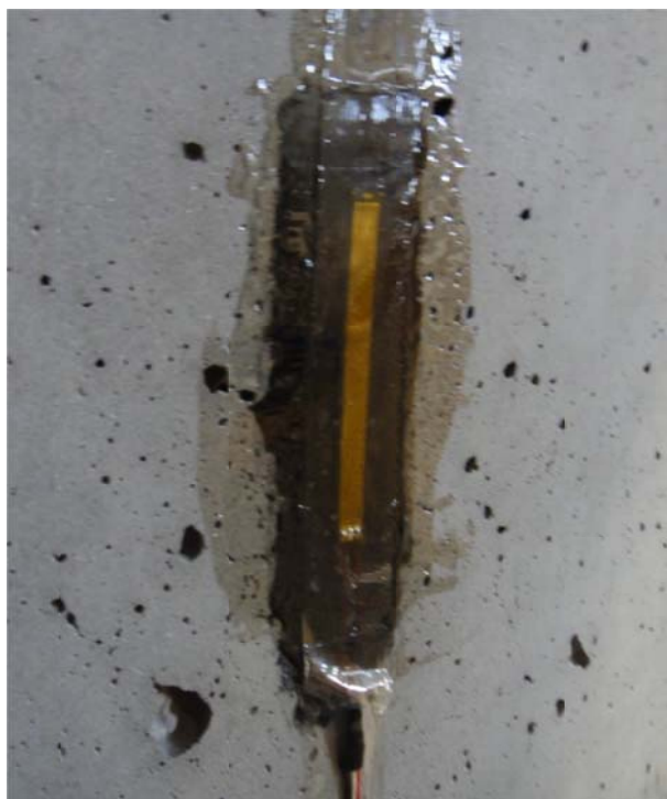
Figure 4-5 Concrete Strain Gage
