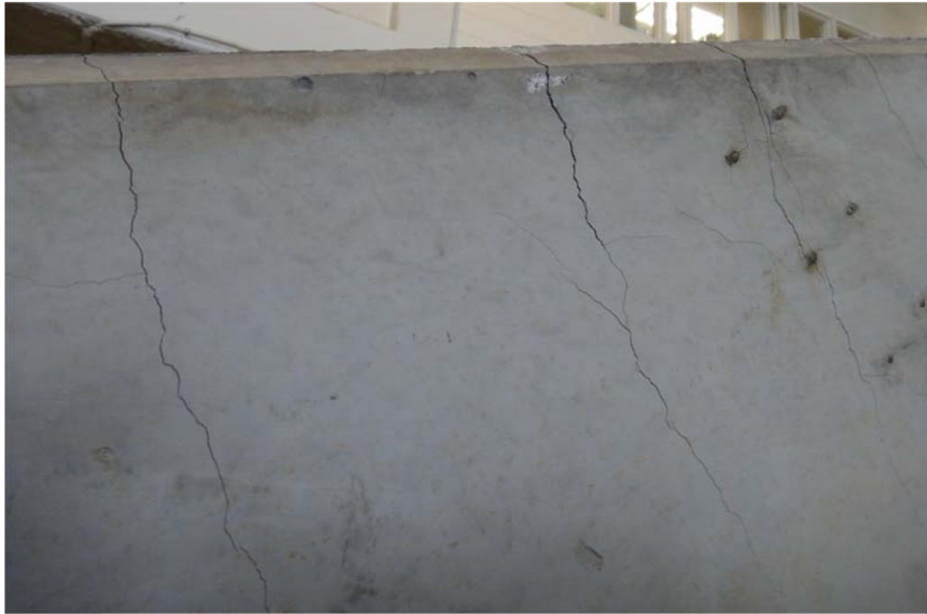
Figure 5-16 Corner Cracks – 144 kips Total Load
