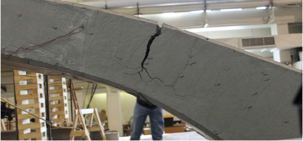
Figure 5-19 Immediately After Failure
