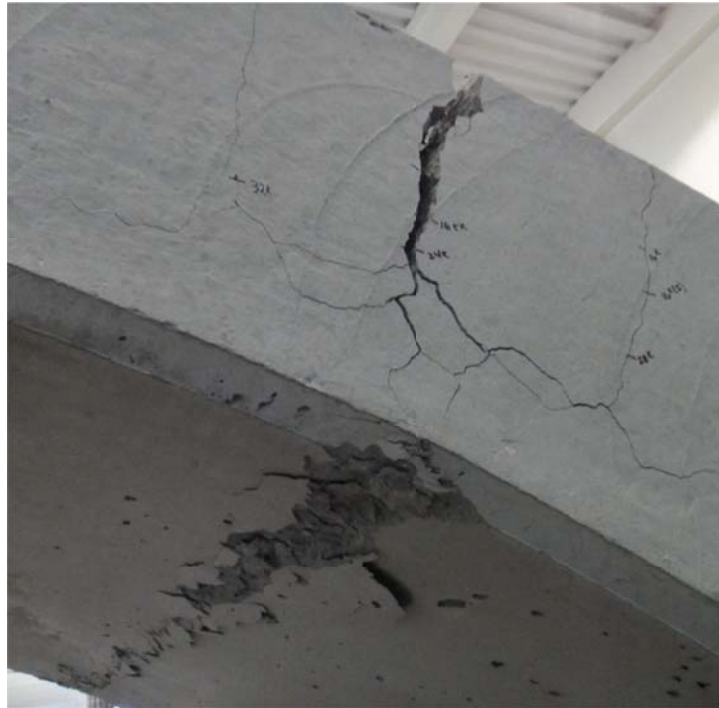
Figure 5-20 Failure Mechanism – Crushed Concrete
