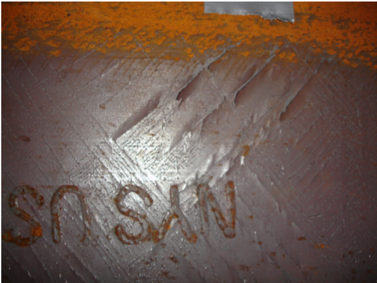
Figure 4.4-3: Striations visible in web of steel section at midspan
