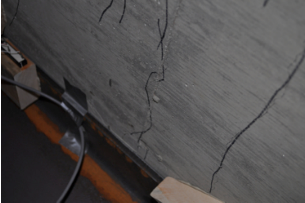
Figure 4.4-10: Cracking in bottom of deck for Specimen 4 after failure
