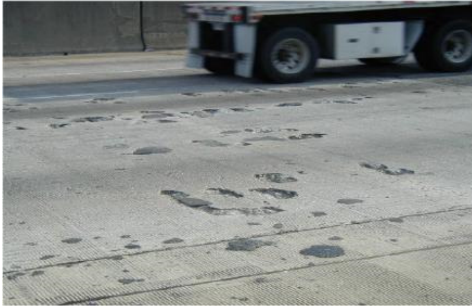
Figure 2.1: Typical Deck Deterioration (Umphrey 2006)
