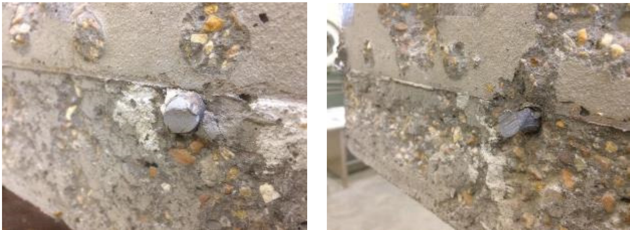
Figure 5.51: SE and SW Reinforcing Steel Failure Condition (R-NEG-F)
