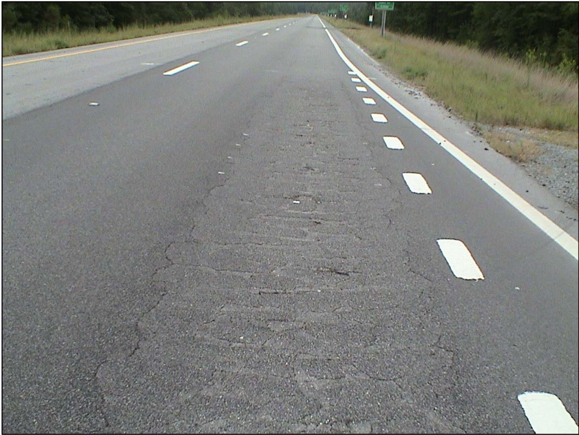
Figure 2.3. Photograph of Fatigue Cracking.
