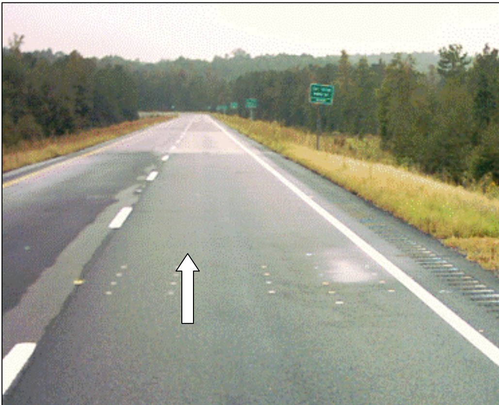
Figure 5.18. Water Ponding Due to Rutting– Section N8.
