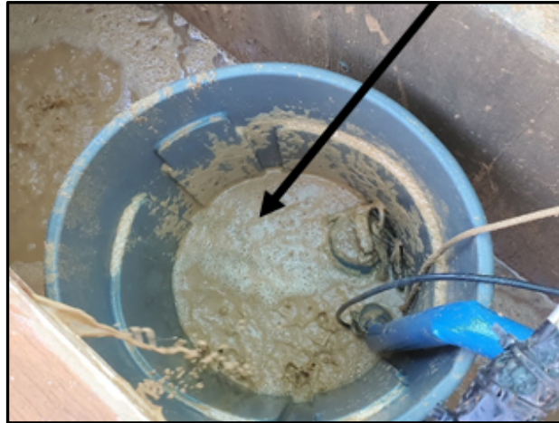
(c) Residue remains after draining runoff
