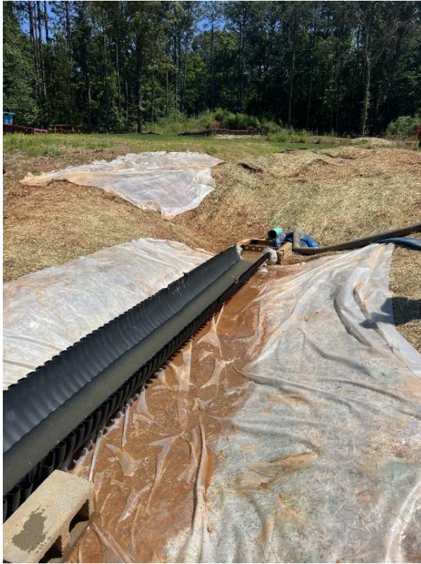
(a) ALDOT underdrain weir box test
