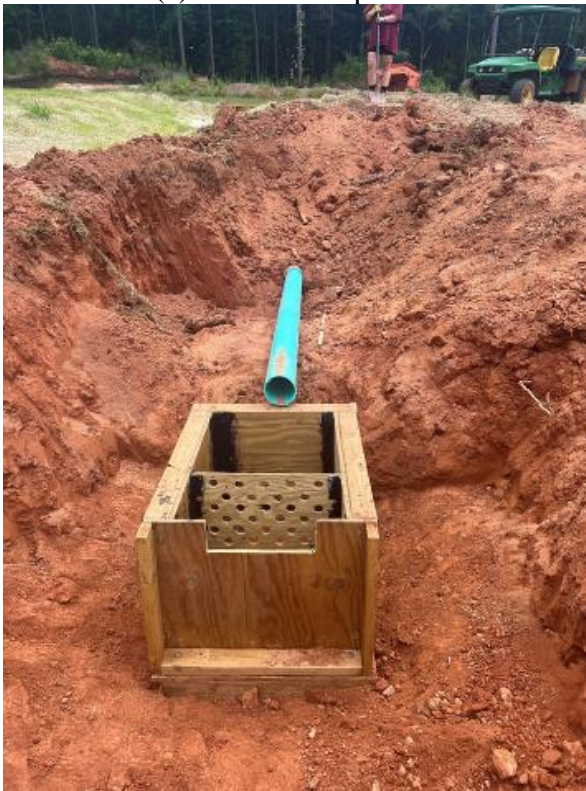
(c) underdrain box
