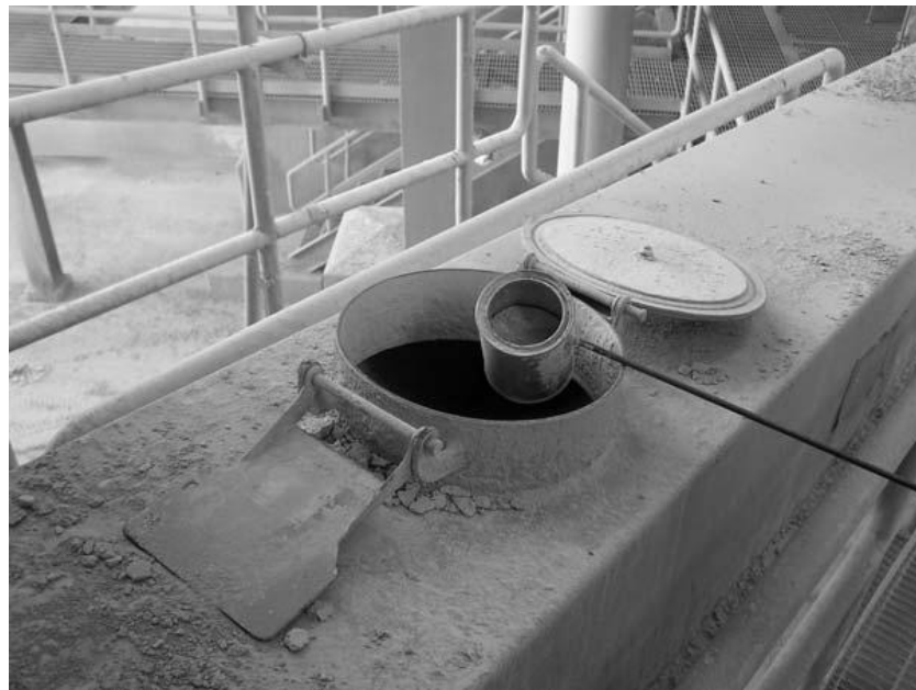
Figure 3.9: Kiln feed sampling point
