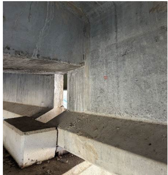
Figure A-4(q): Staining at closed joint edge beam at Bent 3
