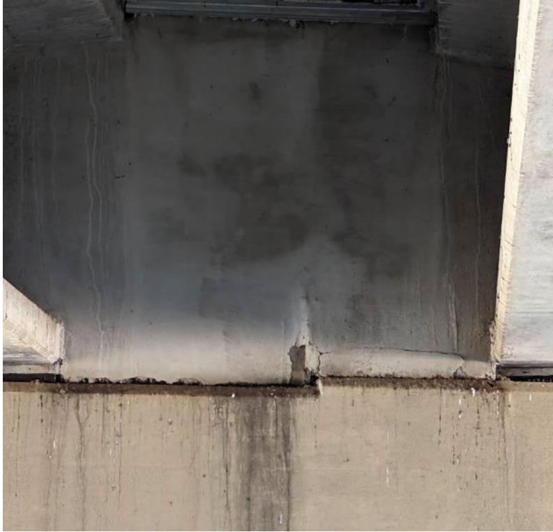
Figure 3-10: Full-depth edge beam with cracking observed (I-20 over Co Rd 49)
