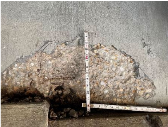
Figure A-5(l): Close-up of more concrete breakout at Bent 3 (Southbound)
