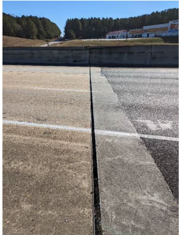
Figure A-4(i): Abutment open joint at Bent 4 (Eastbound)
