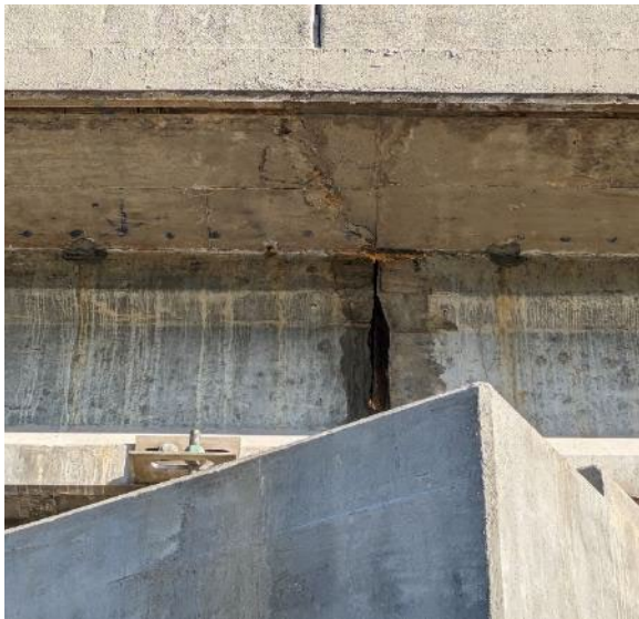
Figure A-1(l): Cracking observed on Northbound side of Bent 2
