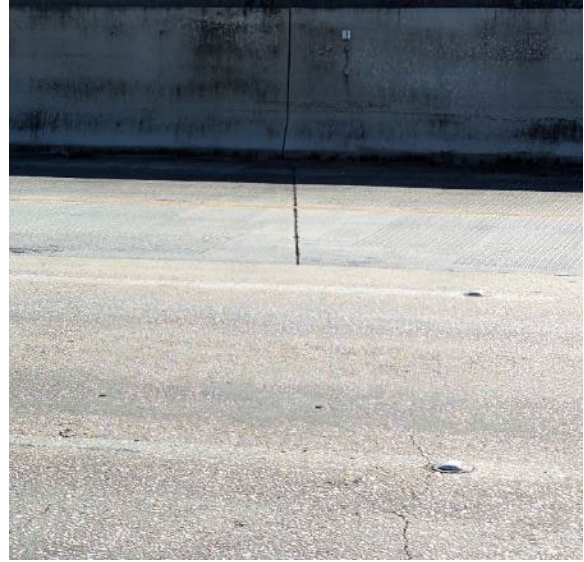
Figure A-4(g): Closed joint at Bent 2 (Eastbound)
