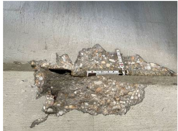
Figure A-5(m): Concrete breakout on Southside at Bent 3 (Southbound)
