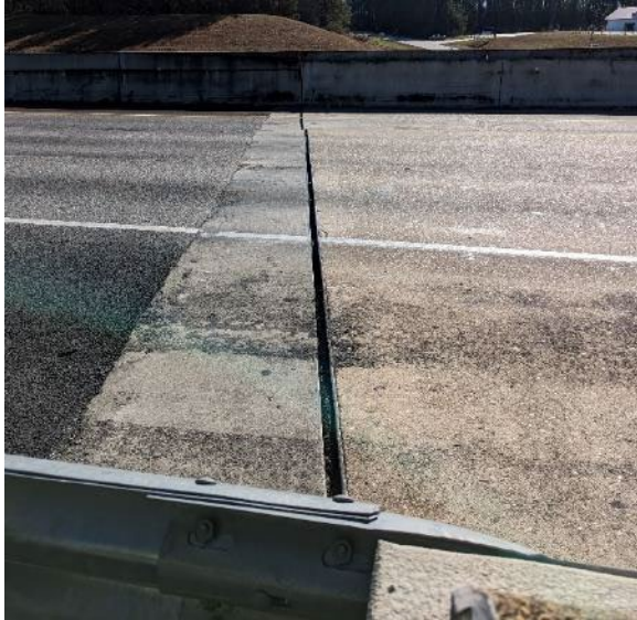
Figure A-4(f): Abutment open joint at Bent 1 (Eastbound)
