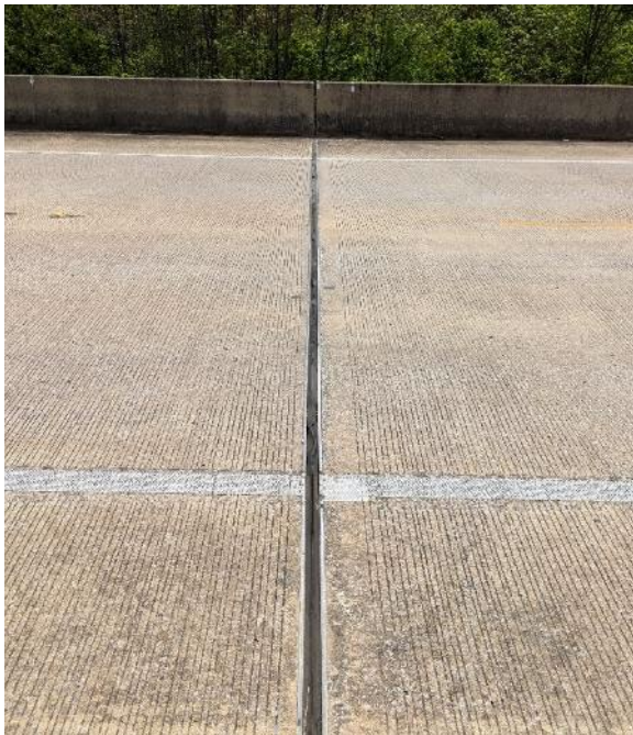
Figure A-6(h): Open joint at Bent 7
