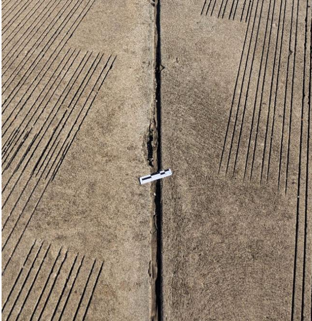
Figure 3-8: Typical spalling observed at closed joint
