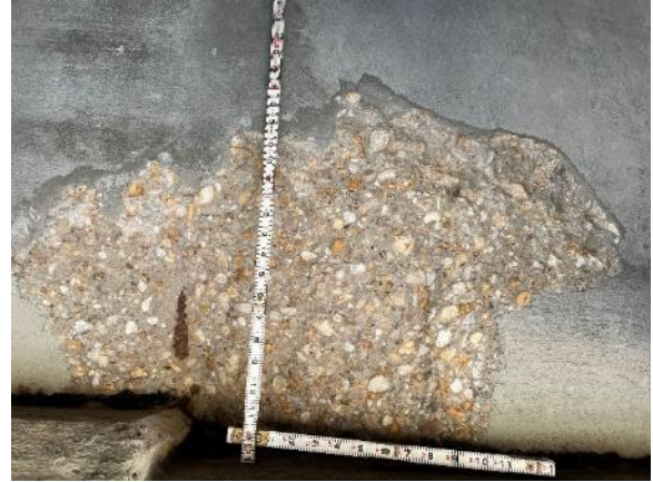
Figure A-5(k): Close-up of concrete breakout at Bent 3 (Southbound)
