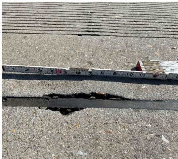
Figure A-5(h): Wearing around sealant on closed joint at Bent 3 (Northbound)
