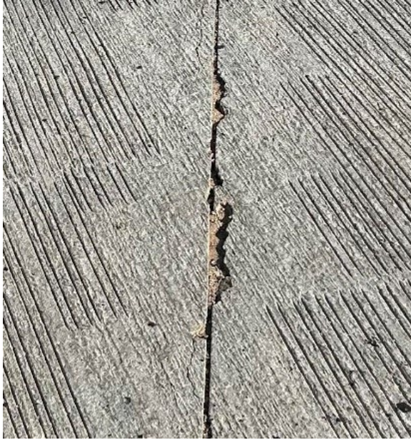
Figure A-2(b): Spalling at closed joint in center stage at Bent 2 (Construction Stage I)
