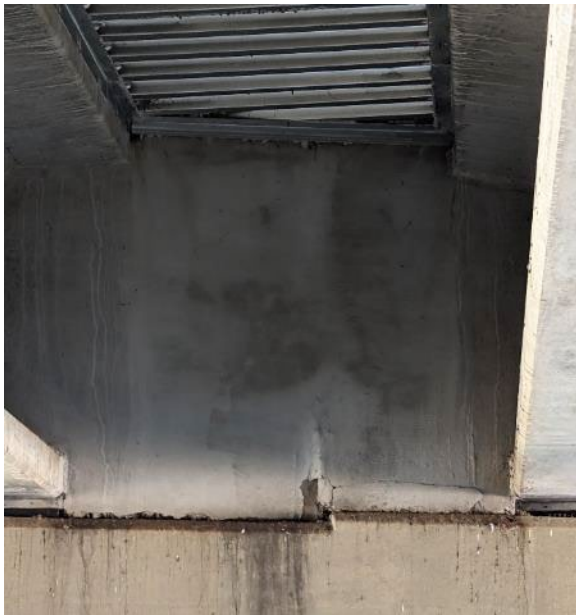
Figure A-4(l): Edge beam at Bent 2 with cracking and staining
