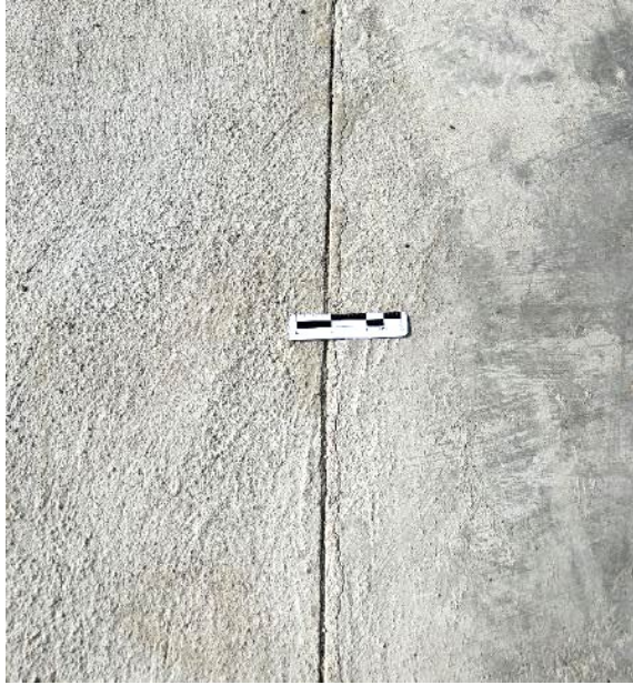
Figure A-2(f): Cracking at closed joint observed at Bent 3 (Construction Stage III)
