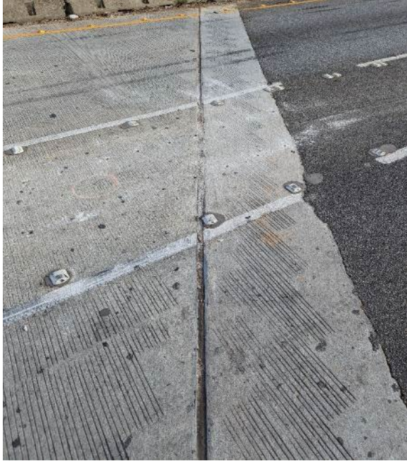
Figure A-1(j): Abutment open joint at Bent 4 (Construction Stage I)
