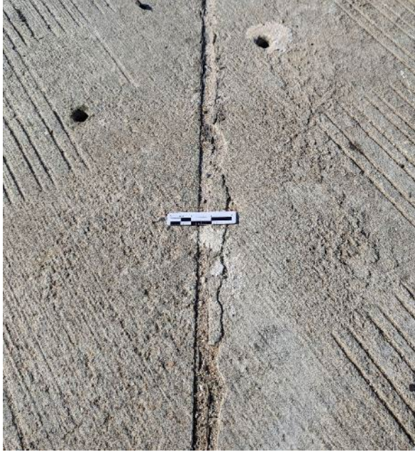
Figure A-1(f): More spalling observed on closed joint at Bent 2 (Construction Stage I)
