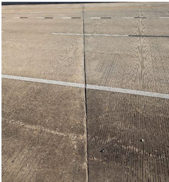
Figure A-3(d): Closed joint at Bent 2
