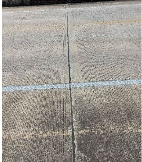
Figure A-6(c): Closed joint at Bent 9
