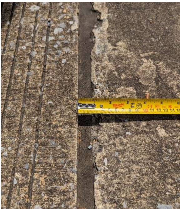
Figure A-6(d): Close-up of closed joint at Bent 9
