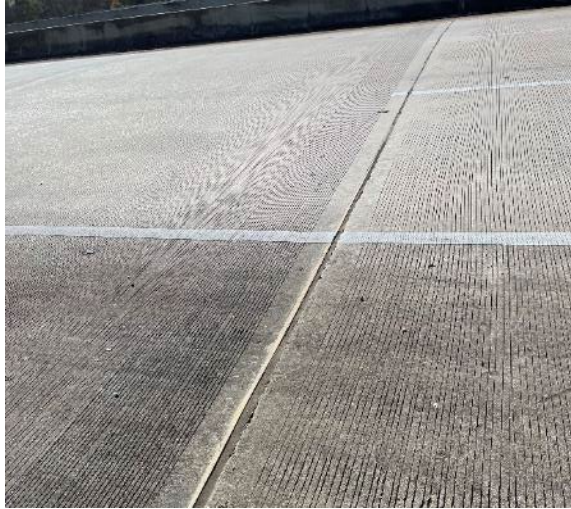
Figure A-5(f): Closed joint at Bent 3 (Northbound)
