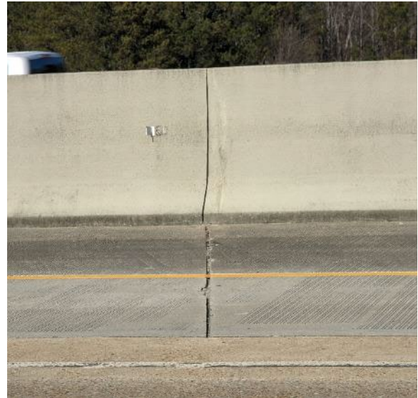
Figure A-4(c): Closed joint at Bent 2 (Westbound)
