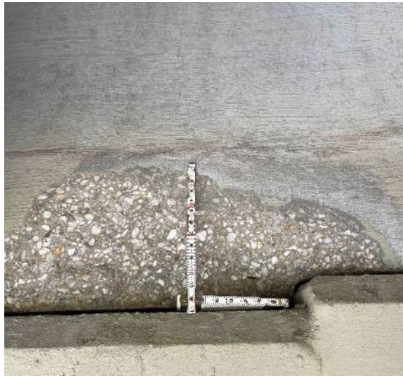
Figure A-5(p): Concrete breakout on edge beam at Bent 3 (Northbound)
