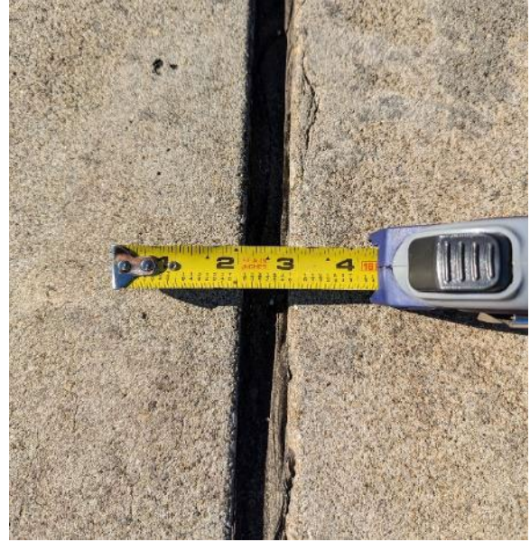
Figure A-3(g): Close-up of spalling observed at closed joint on Bent 2
