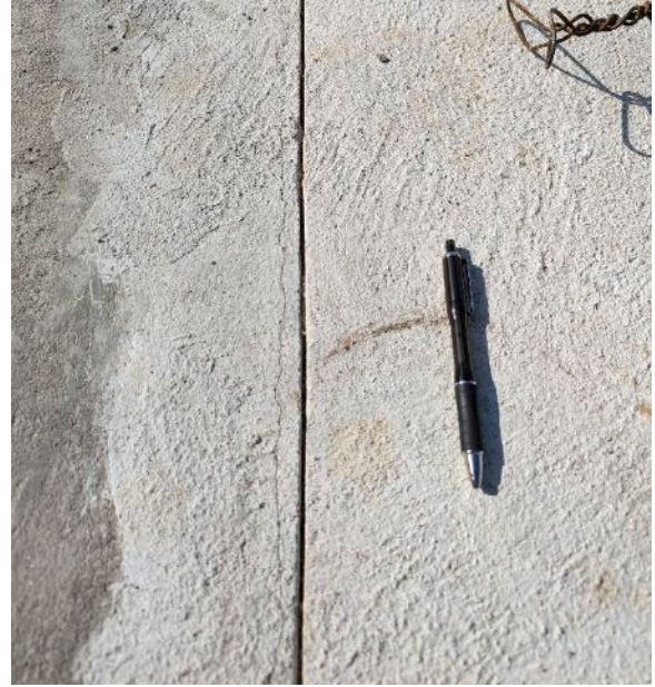
Figure A-2(c): Cracking at closed joint observed at Bent 2 (Construction Stage III)
