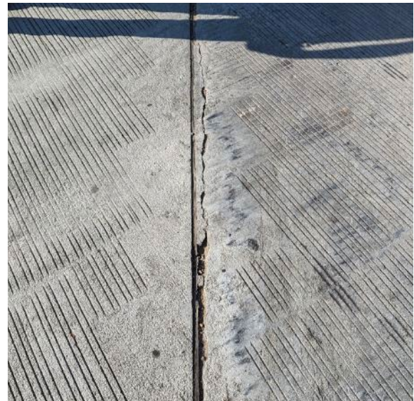
Figure A-1(e): Cracking and spalling observed on closed joint at Bent 2 (Construction Stage I)
