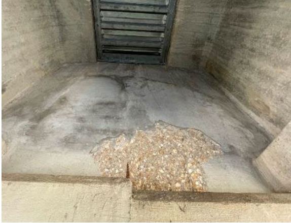
Figure A-5(j): Concrete breakout on Northside of Bent 3 (Southbound)
