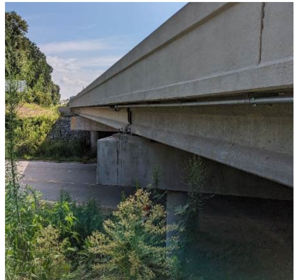
Figure A-1(m): Leakage observed on Southbound side of Bent 2
