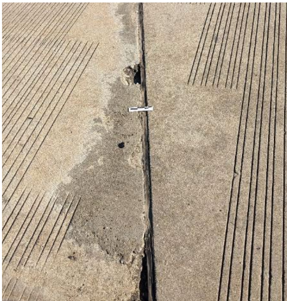
Figure A-3(h): More spalling observed at closed joint on Bent 2
