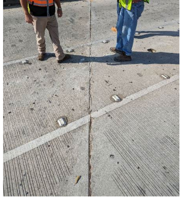
Figure A-1(g): Closed joint at Bent 3 (Construction Stage I)
