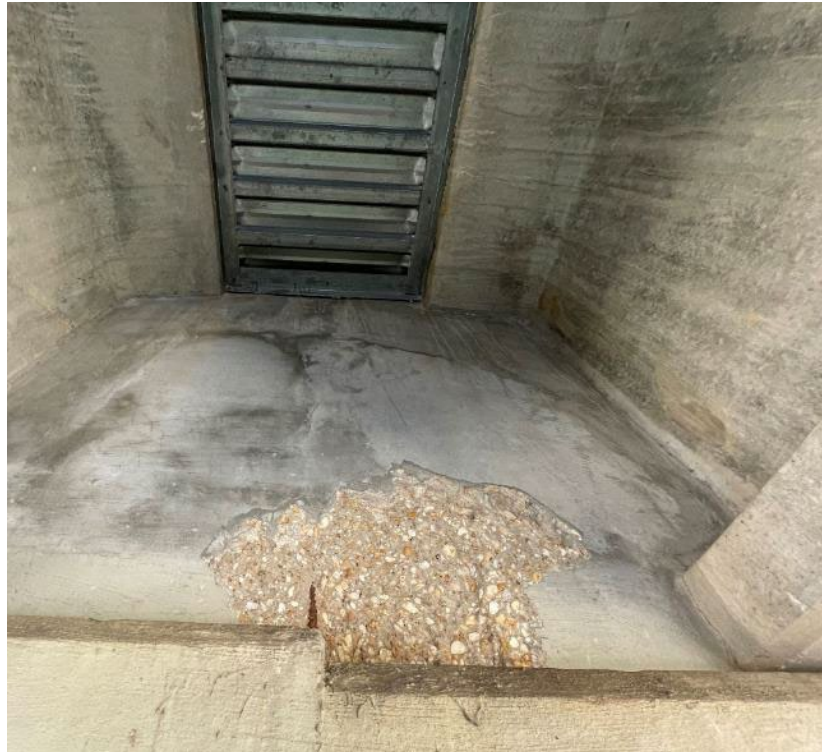
Figure 3-11: Full-depth edge beam with significant concrete breakout (Co Rd 39 over I-10)
