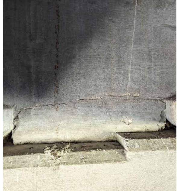
Figure A-3(k): Cracking in edge beam at closed joint
