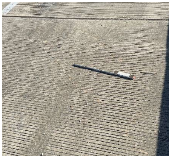
Figure A-5(d): Long hairline cracks on closed joint at Bent 3 (Southbound)
