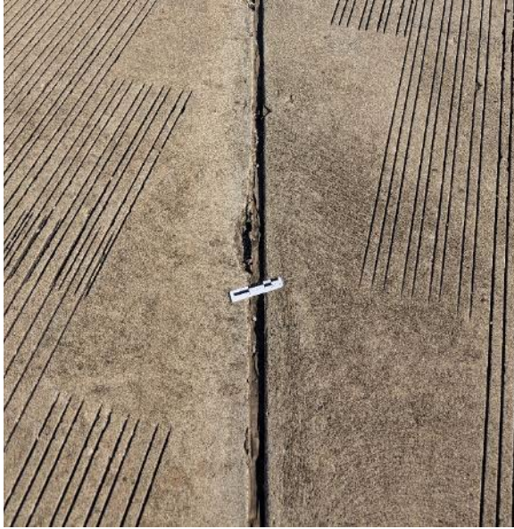
Figure A-3(f): Spalling observed at closed joint on Bent 2
