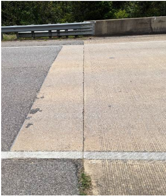
Figure A-6(b): Open joint at north abutment
