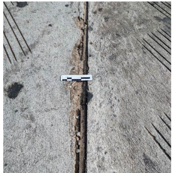
Figure A-1(i): Spalling observed on open joint at Bent 3 (Construction Stage I)
