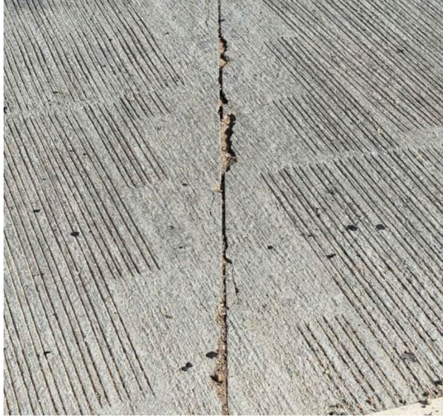
Figure 3-9: Spalling and cracking observed at the freshly constructed closed joint (LEE-2)
