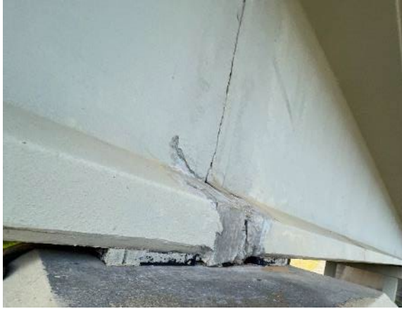
Figure A-5(n): Westside of closed joint on Bent 3 (Southbound)
