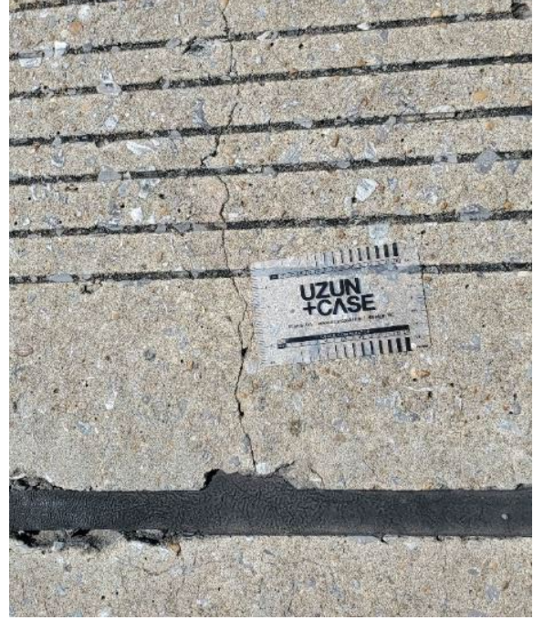
Figure A-6(g): Crack observed on closed joint at Bent 8
