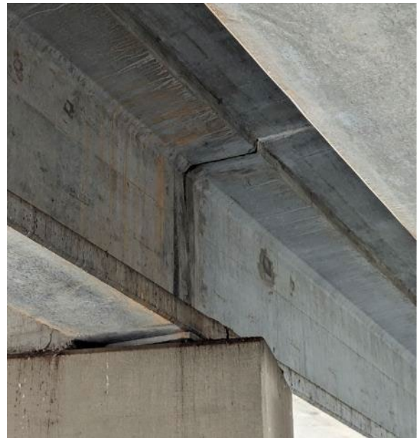
Figure A-4(m): Closed joint on the underside of bridge at Bent 2
