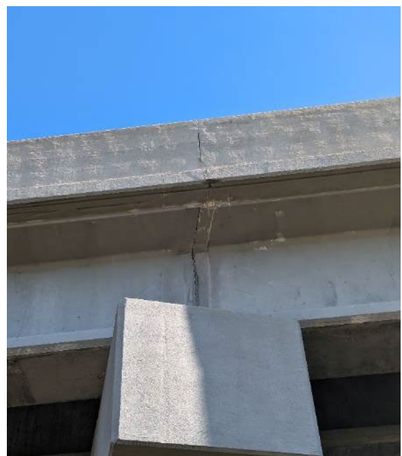
Figure A-3(m): Staining on Southside of closed joint
