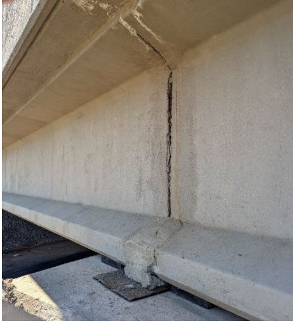
Figure A-3(j): Staining observed on Northside of closed joint
