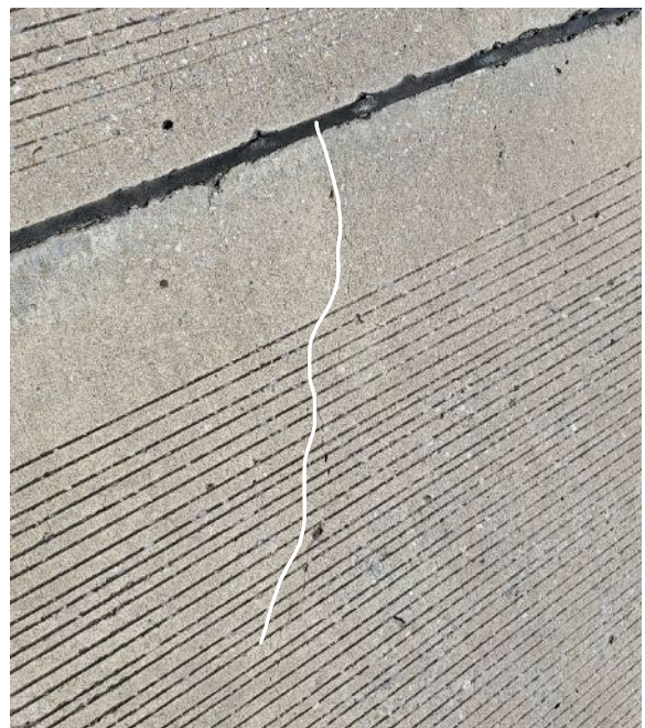
Figure A-6(e): Crack observed on closed joint at Bent 9
