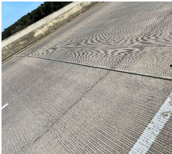
Figure A-5(b): Closed joint at Bent 3 (Southbound)
