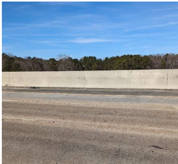
Figure A-4(d): Closed joint at Bent 3 (Westbound)
