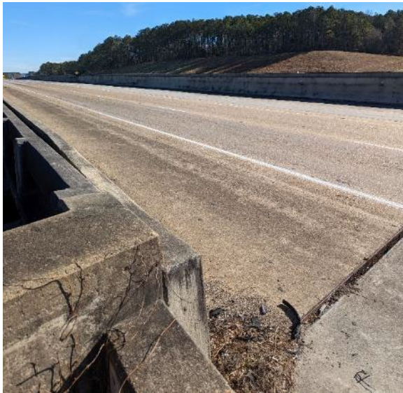
Figure A-4(b): Abutment open joint at Bent 1 (Westbound)
