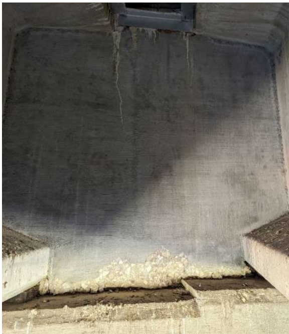
Figure A-3(l): Concrete breakout and staining on edge beam for Bent 2
