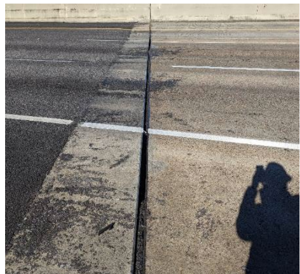
Figure A-4(e): Abutment open joint at Bent 4 (Westbound)
