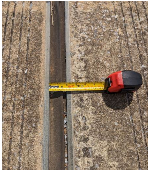
Figure A-6(i): Closeup of open joint at Bent 7
