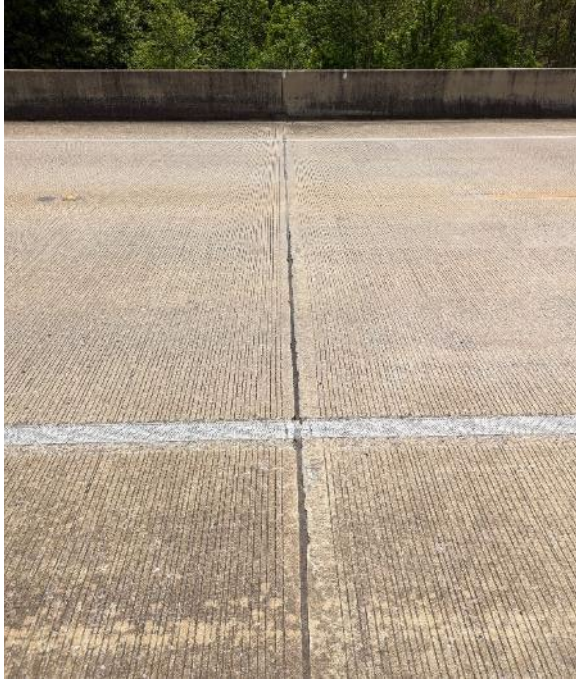
Figure A-6(f): Closed joint at Bent 8
