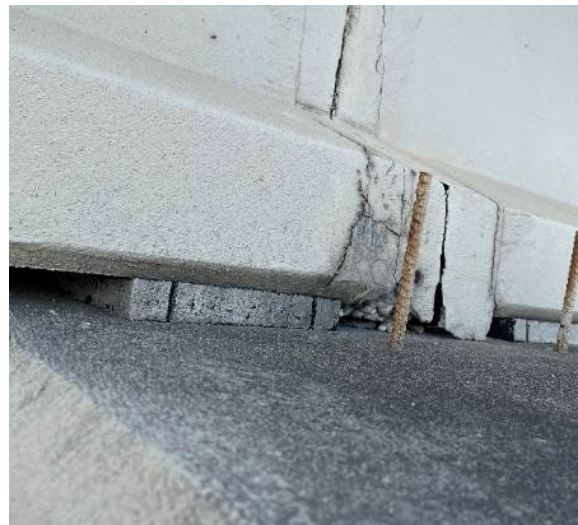
Figure A-5(q): Exposed rebar on Eastside closed joint (Northbound)
