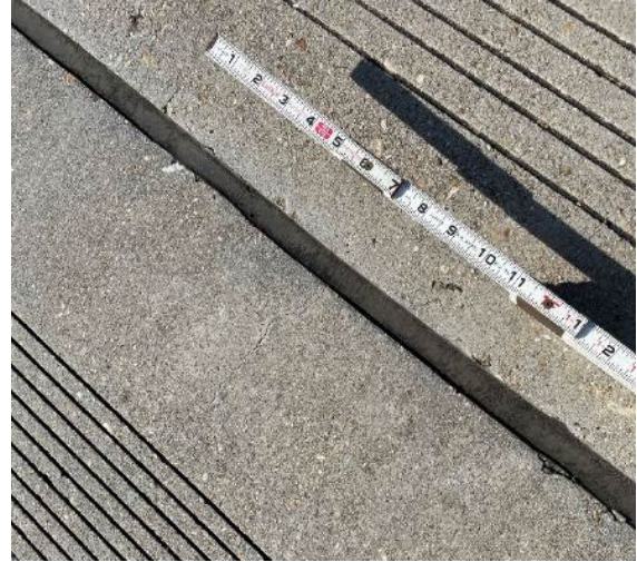
Figure A-5(g): Hairline cracks observed on closed joint at Bent 3 (Northbound)
