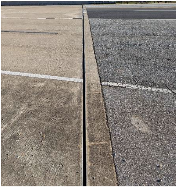
Figure A-3(b): Abutment open joint at Bent 1
