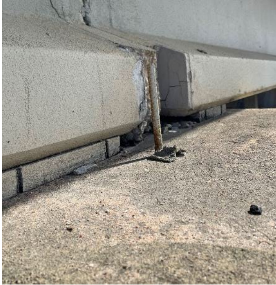
Figure A-5(r): Exposed rebar on westside closed joint (Northbound)
