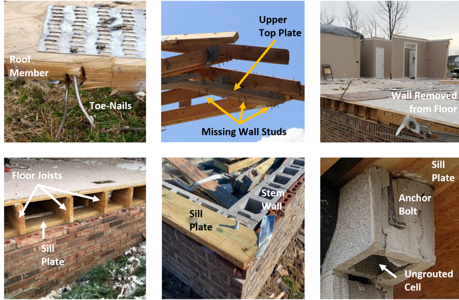
Figure 2.2. Various load path failures observed during field surveys.
