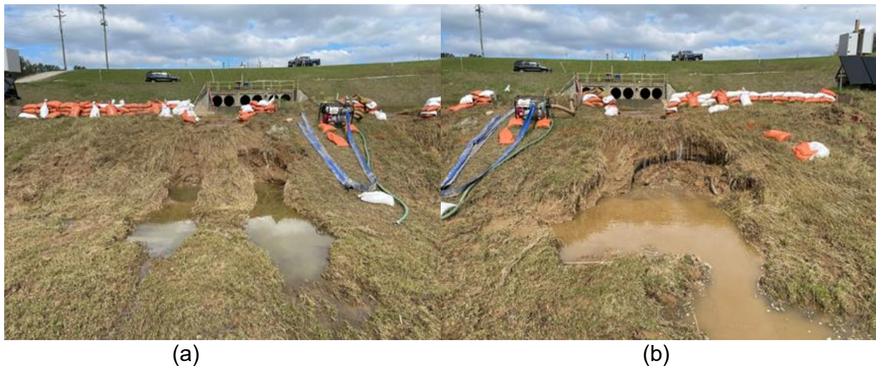
Figure 10. Post-overtopping condition of the embankment, illustrating the treated (a) and untreated (b) sections.
