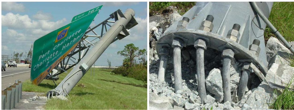
Figure 1-3. Sign Support Structure Failure at the I-75 and SR 17 Interchange, Florida, Due to Hurricane Charley in 2004 (Faquir et al., 2005).
