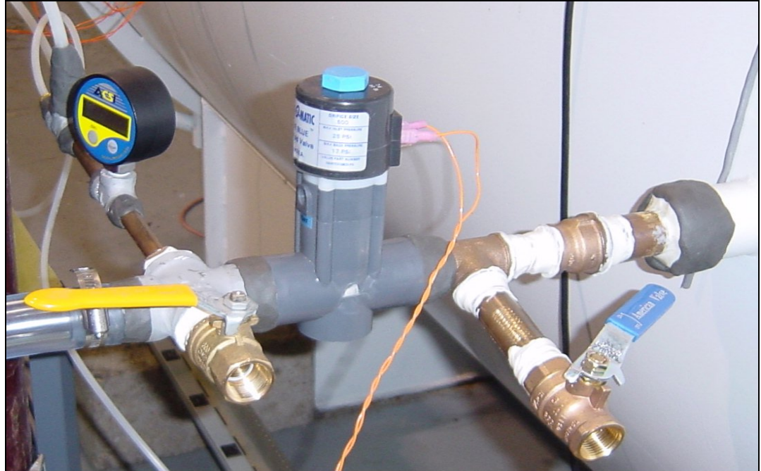
Figure 13: Solenoid Used to Pulse Gas to the Manifold
