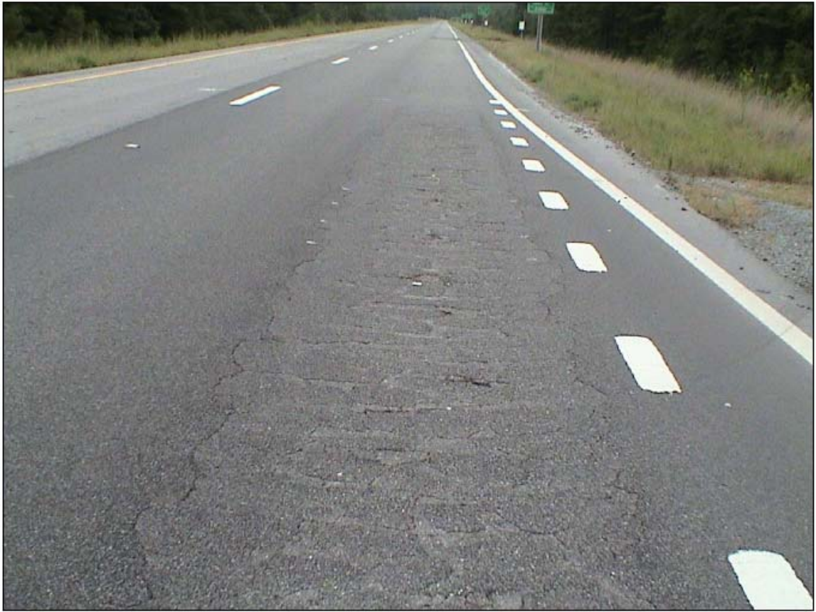
Figure 1-2. Fatigue Cracking on a Roadway (Priest and Timm, 2006).
