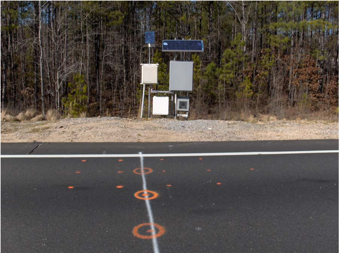
Figure 6-7. Remote Roadside Boxes.
