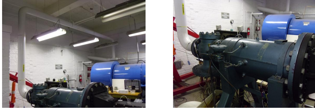
Figure 24: Compressed Air Supply Line Pipe and Stagnation/Settling Chamber
