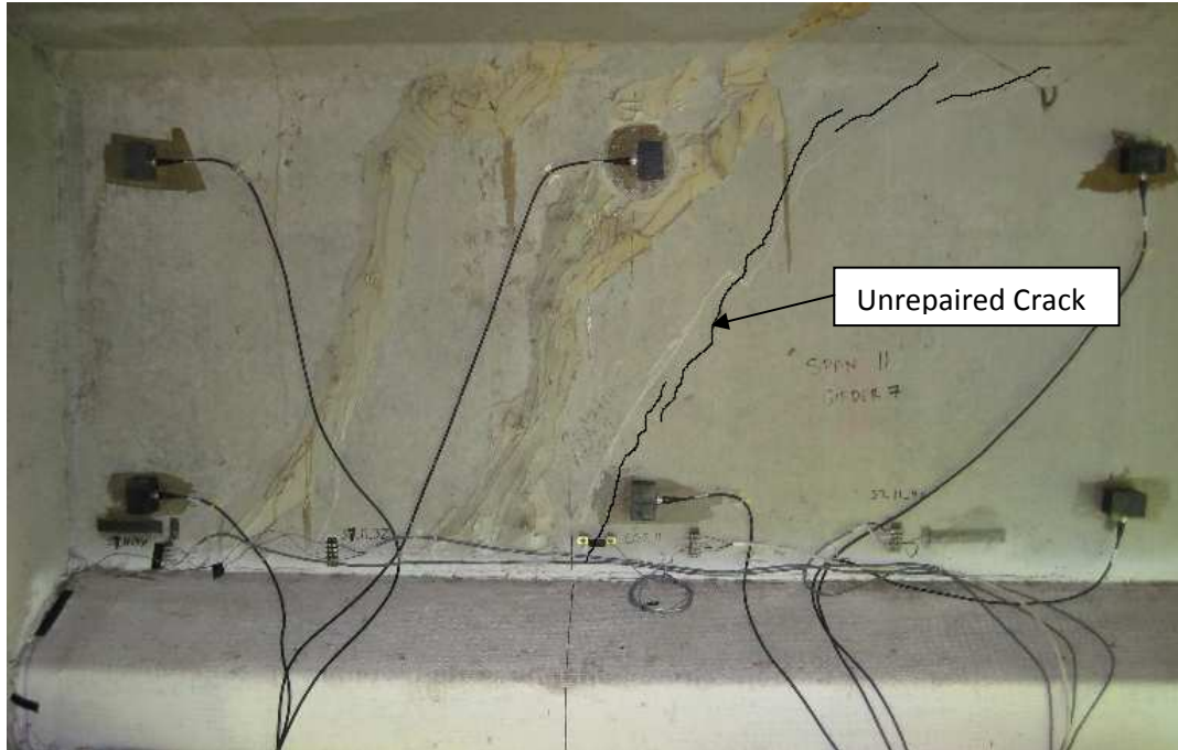
Figure 5-30: Visible cracks on face of SP11G7
