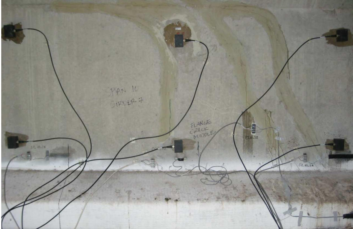
Figure D-3: Visible cracks on face of SP10G7
