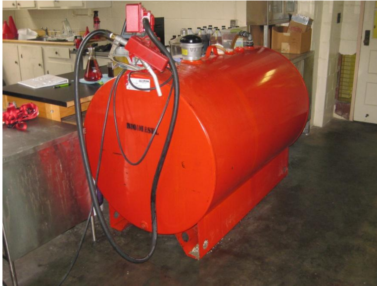
Figure 3.8. Storage tank for processed biodiesel.
