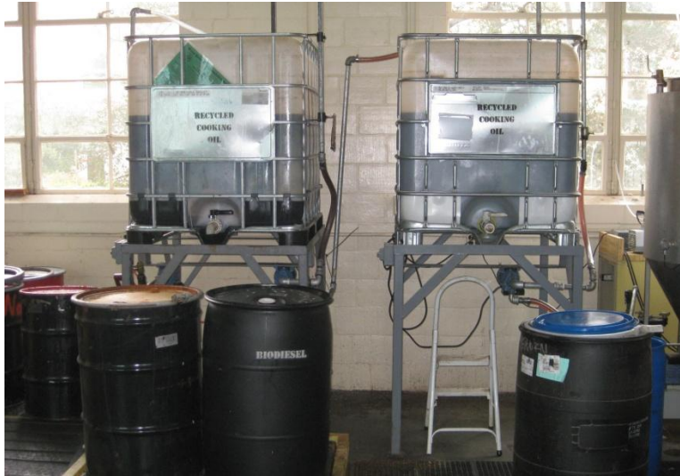
Figure 3.7. Primary (left) and secondary (right) WVO settling tanks.
