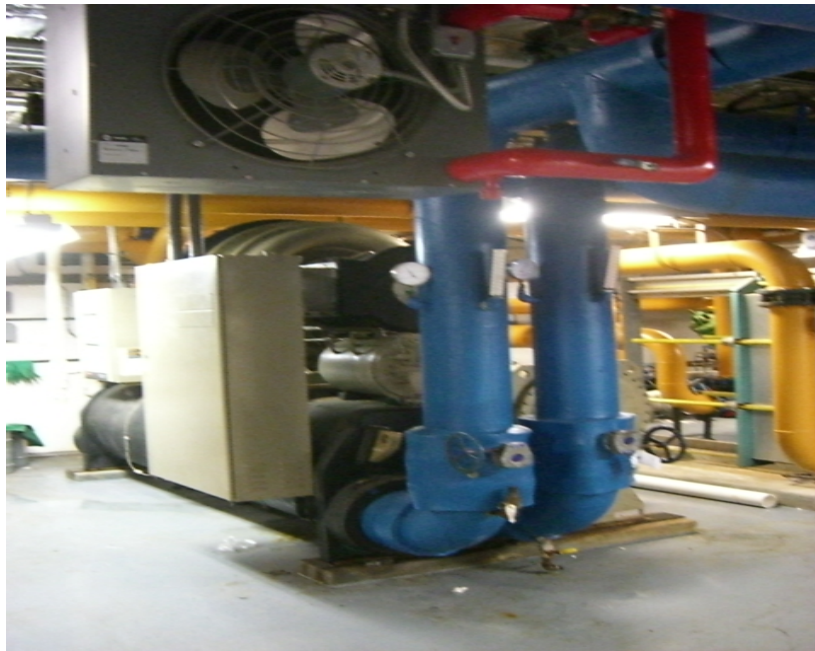
Figure 4.6 RMC Chiller Photo
