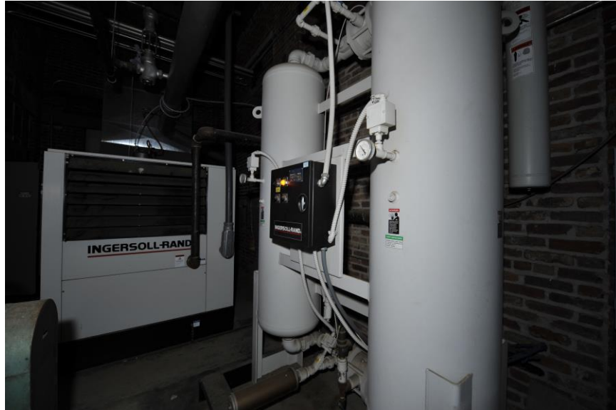
Figure 21: Ingersoll Rand HRD45-FHSC Compressed Air Dryer
