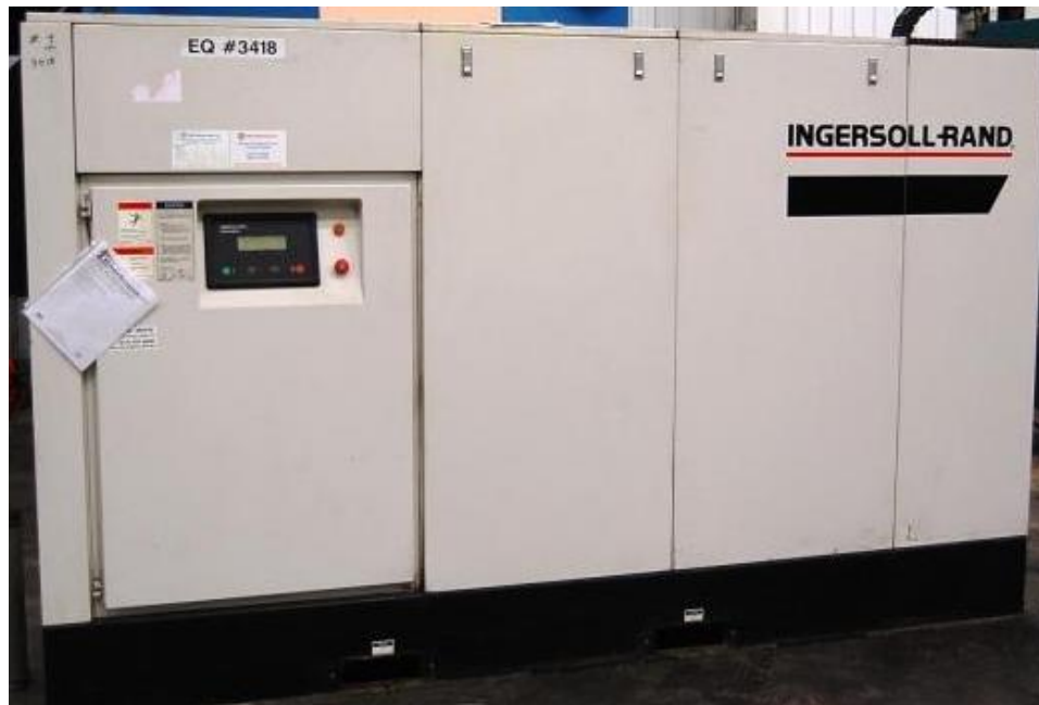
Figure 20: Ingersoll Rand SSR-EP150 Compressor
