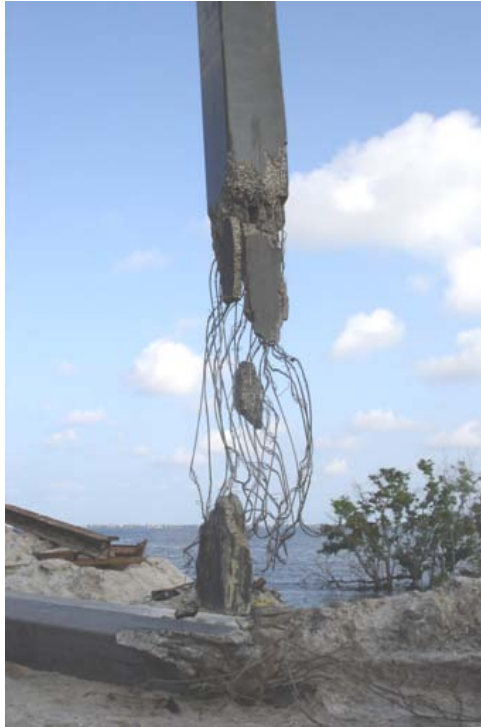
Figure 2.19. Damaged PCPS pile (adapted from Likins 2011)
