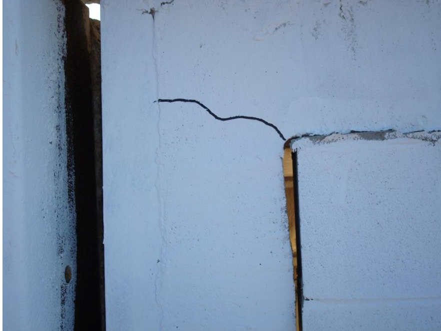
Figure 3.39: Support Cracking of Wall 1
