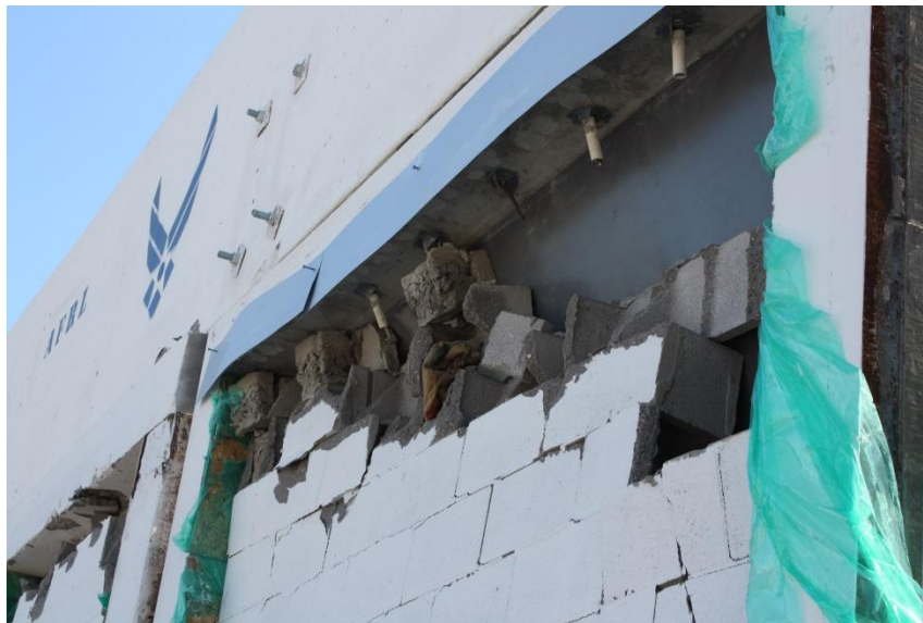
Figure 6.14: Post Test Exterior View
