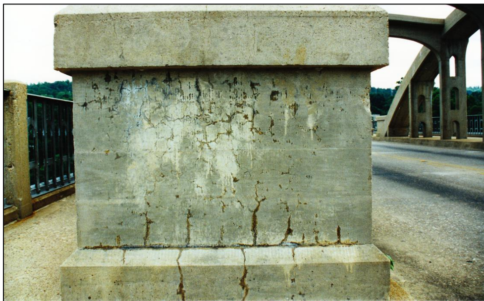
Figure 3.23. Map-cracking on an abutment of span 5
