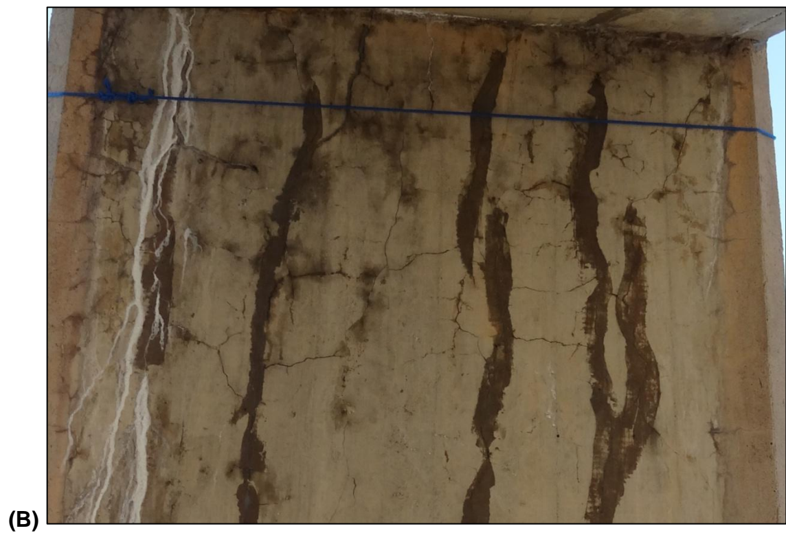
Figure 6.14. Additional cracking in span 5 – north arch, (A) November 2010 and (B) August 2013
