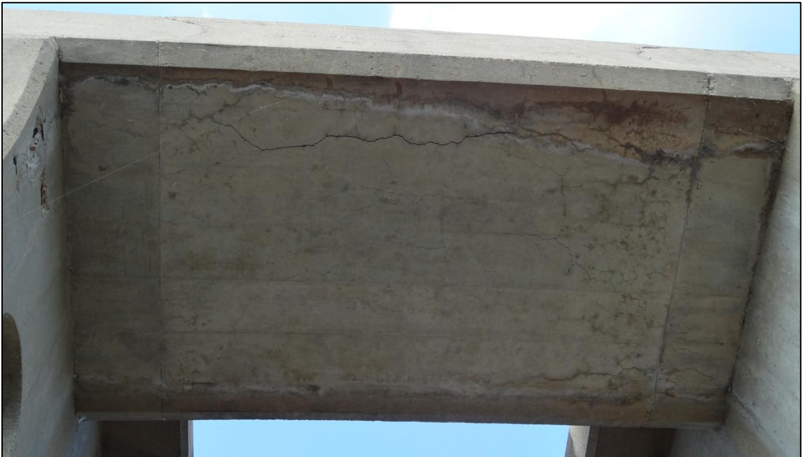
Figure 7.11. Examples of possible ASR in span 4
