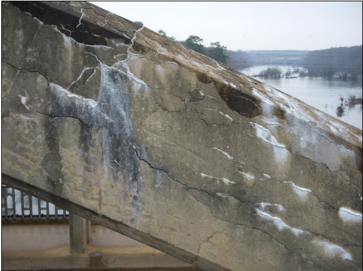
Figure 3.16. Severe distress due to ASR on span 5, south arch
