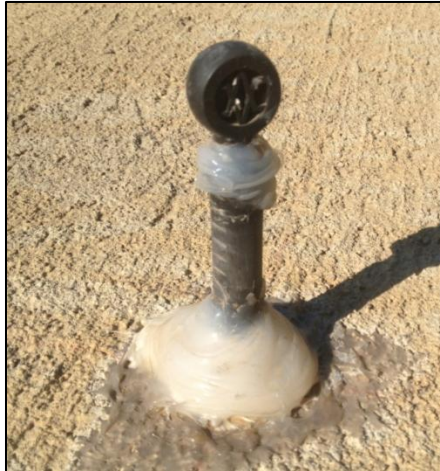
Figure 5.4. Plastic tube with rubber plug installed in concrete
