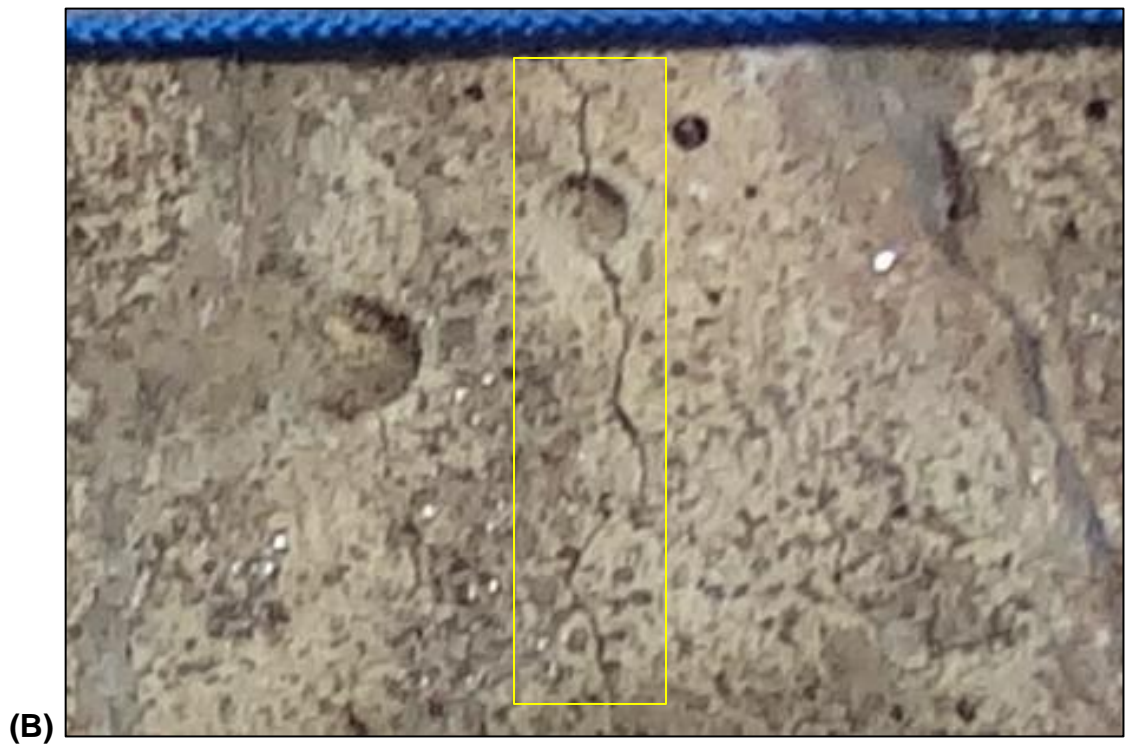
Figure 6.15. Crack widening on span 5 – south arch, (A) November 2010 and (B) August 2013
