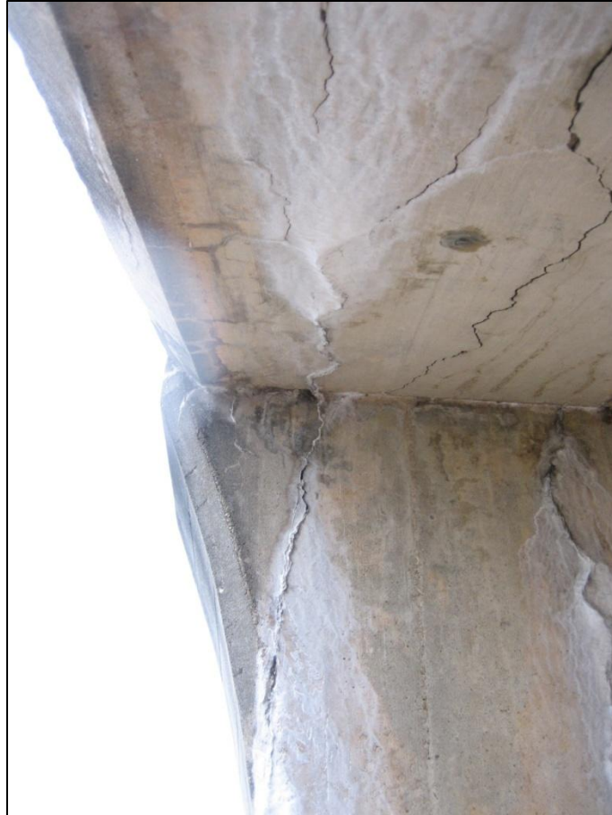
Figure 3.22. Cracking and surface deposits extending from arch to hanger
