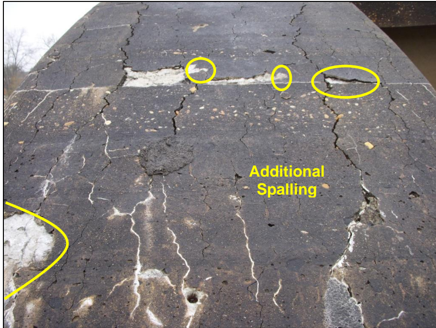
Figure 3.19. Additional spalling on span 5 south from 3/11/08 to 12/14/09
