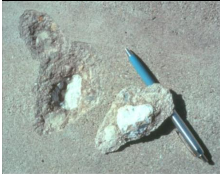
Figure 2.6. Concrete popout caused by ASR (Fournier et al. 2004)
