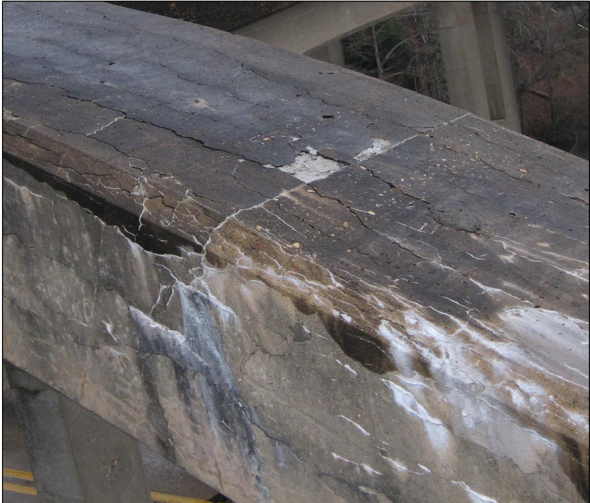
Figure 1.2. Surface deposits and ASR-induced cracking on 3/11/08
