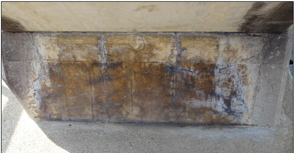
Figure 7.10. Examples of possible ASR in span 3
