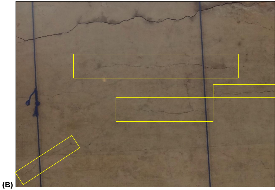
Figure 6.13. Widening and elongation of existing cracks in span 4 – south arch, (A) November 2010 and (B) August 2013
