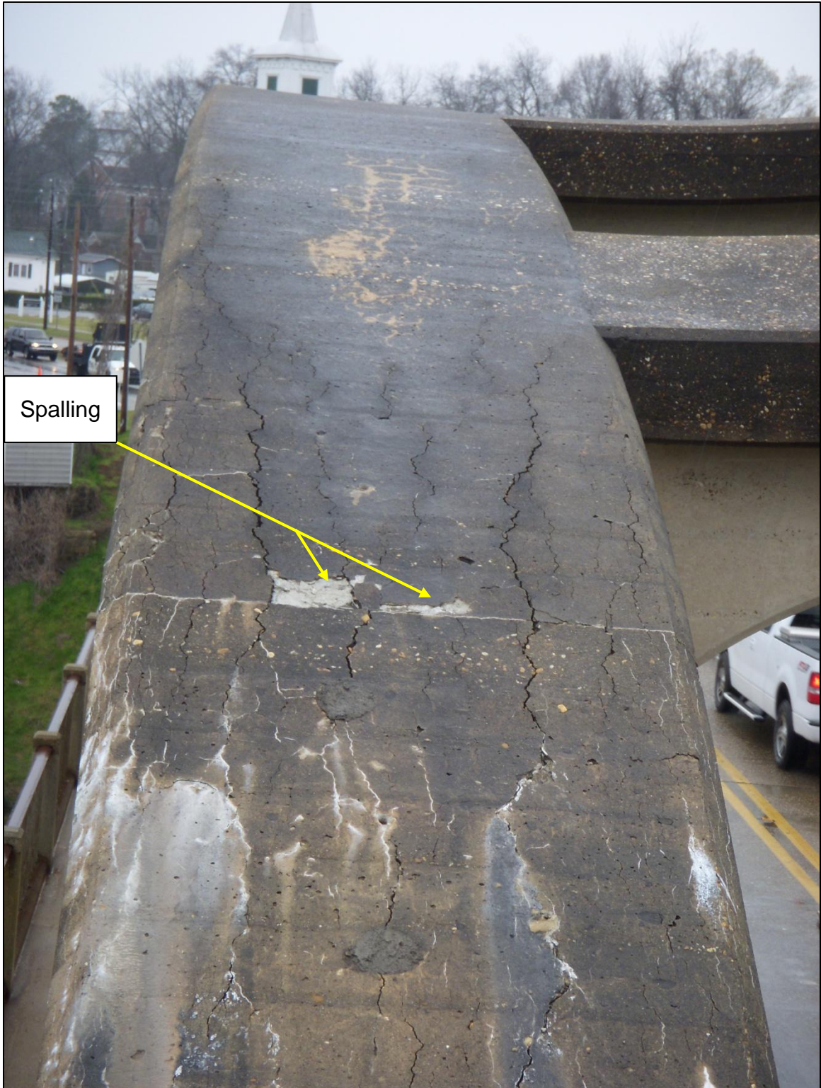
Figure 3.18. Closer view of longitudinal cracking and spalling on span 5 south on
