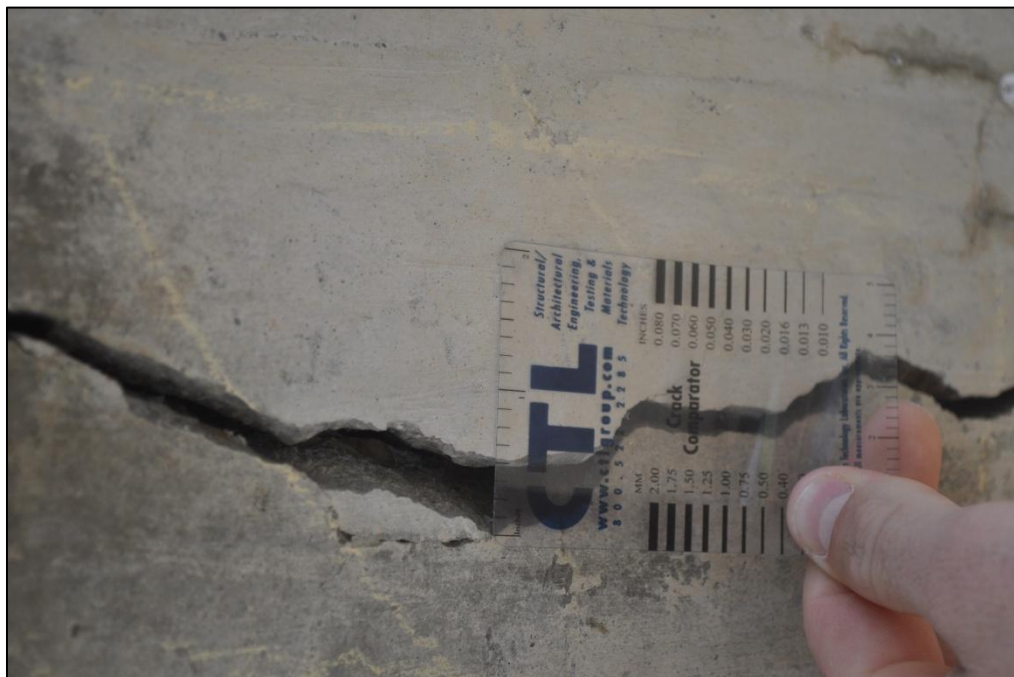
Figure 3.20. Crack width close to 1/2 inch
