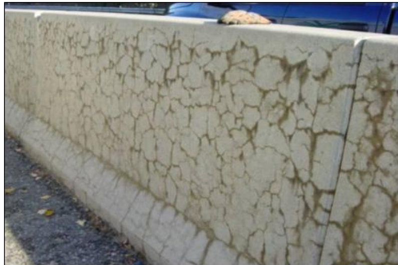
Figure 2.3. Severe map-cracking and surface discoloration on a road barrier (Fournier et al. 2010)
