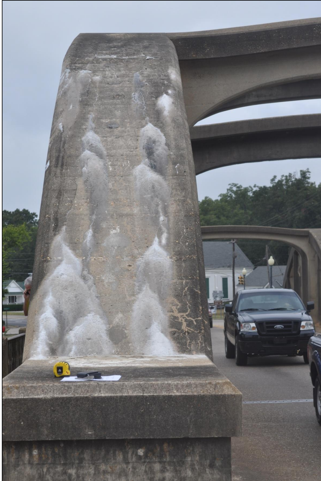
Figure 3.17. Distress with surface deposits of efflorescence and alkali-silica gel on the eastern side of span 5 south
