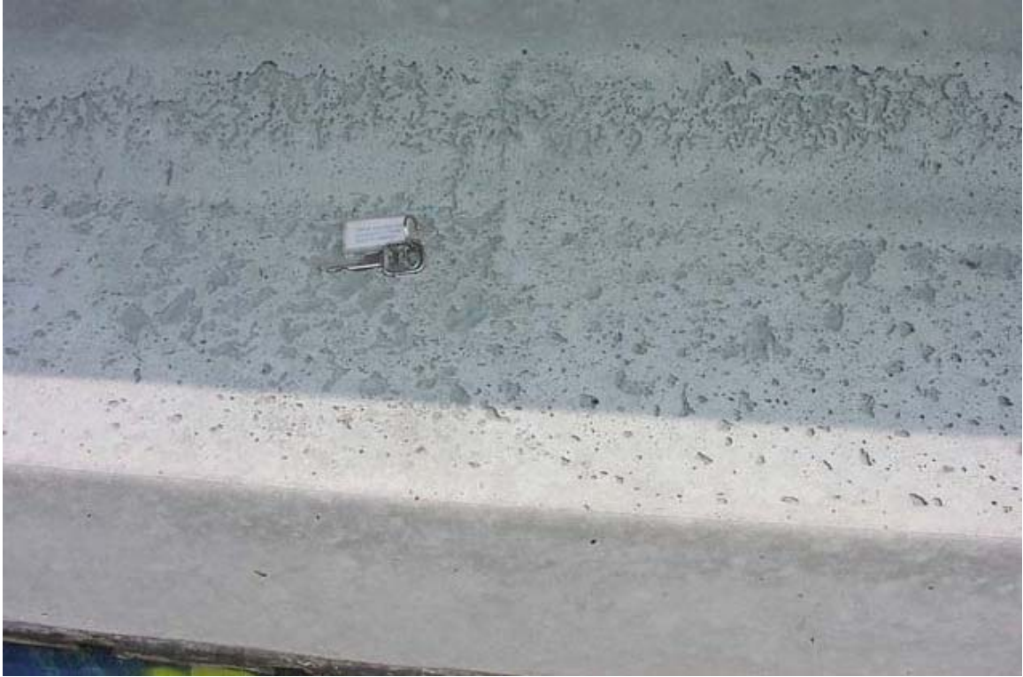
Figure 3.2: Shallow bugholes along upper surface of bottom flange, where pooling bleedwater was trapped against the formwork (Ozyildirim 2008)
