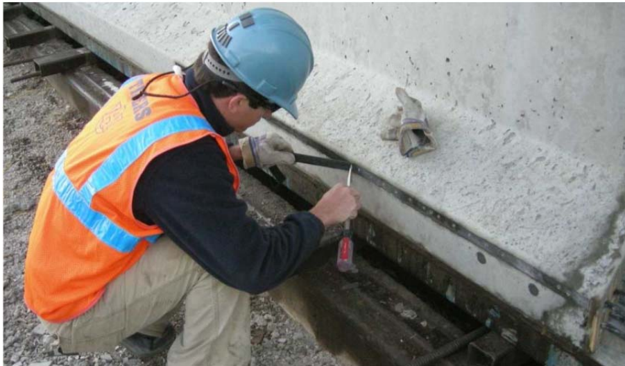
Figure 4.1: Installation of DEMEC mounting strips ( top ) before closure of formwork and ( bottom ) following removal of formwork
