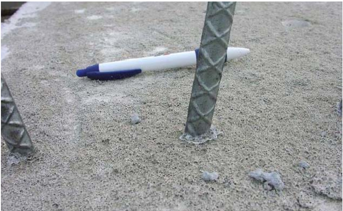
Figure 3.3: Frothy, deleterious material that collected on the top surface of girders cast with high-slump-flow SCC of questionable stability (Ozyildirim 2008)
