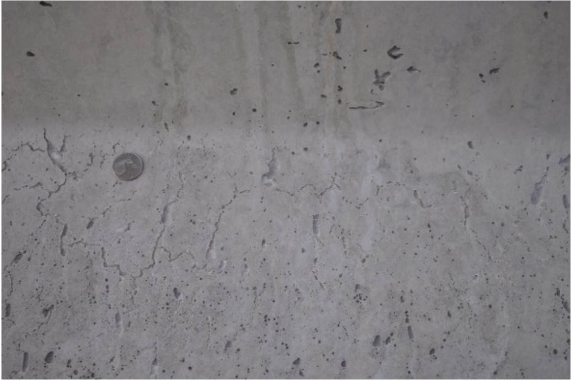
Figure 3.22: Shallow bleed channels in SCC girder (U.S. quarter for scale)
