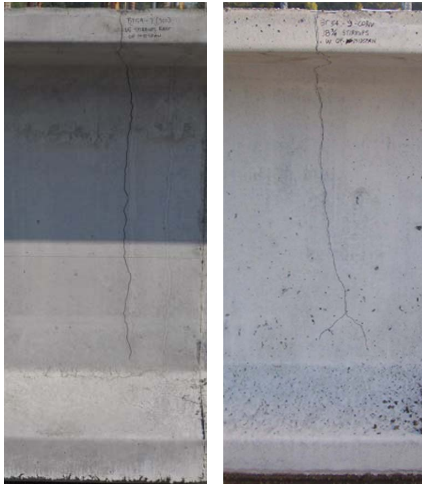
Figure 3.21: Cracking of girders constructed with ( left ) SCC and ( right ) VC
