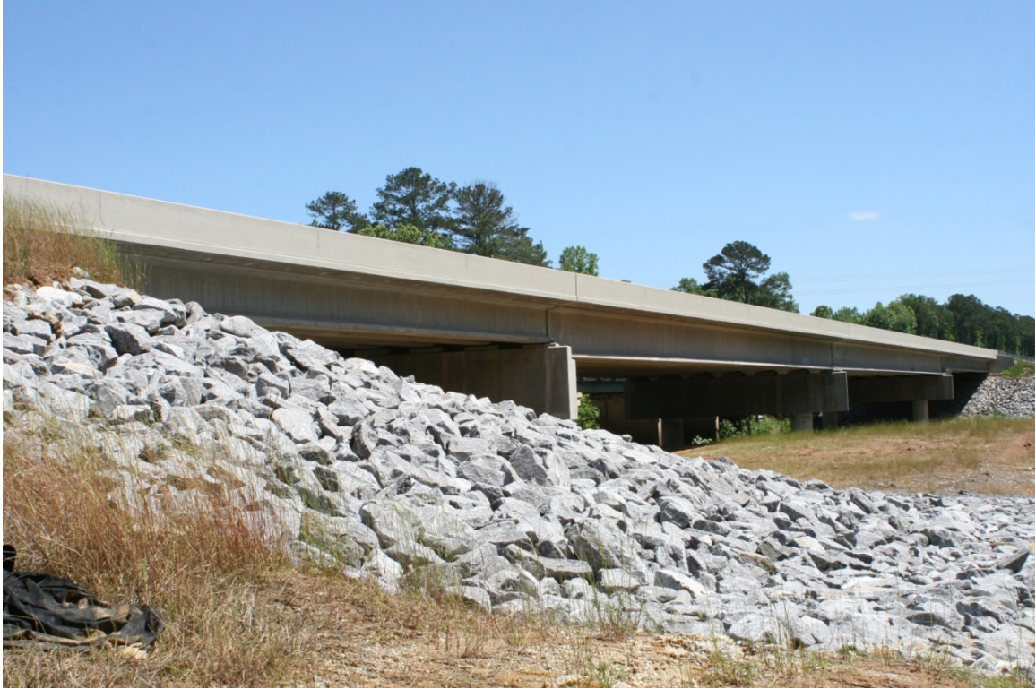
Figure 3.1: Completed bridge over Hillabee Creek (left two spans are SCC girder spans)
