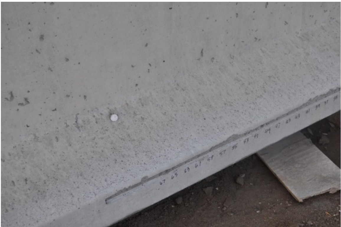
Figure 3.23: Shallow surface flaws in SCC girder (U.S. quarter for scale)
