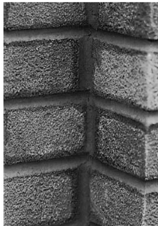
A-5-3 The correct way to finish a corner (The Brick Development Association 2005)
