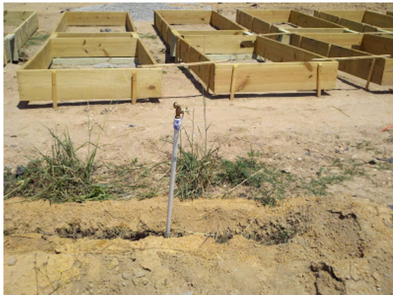
Figure 5. Plumbing in the site.
