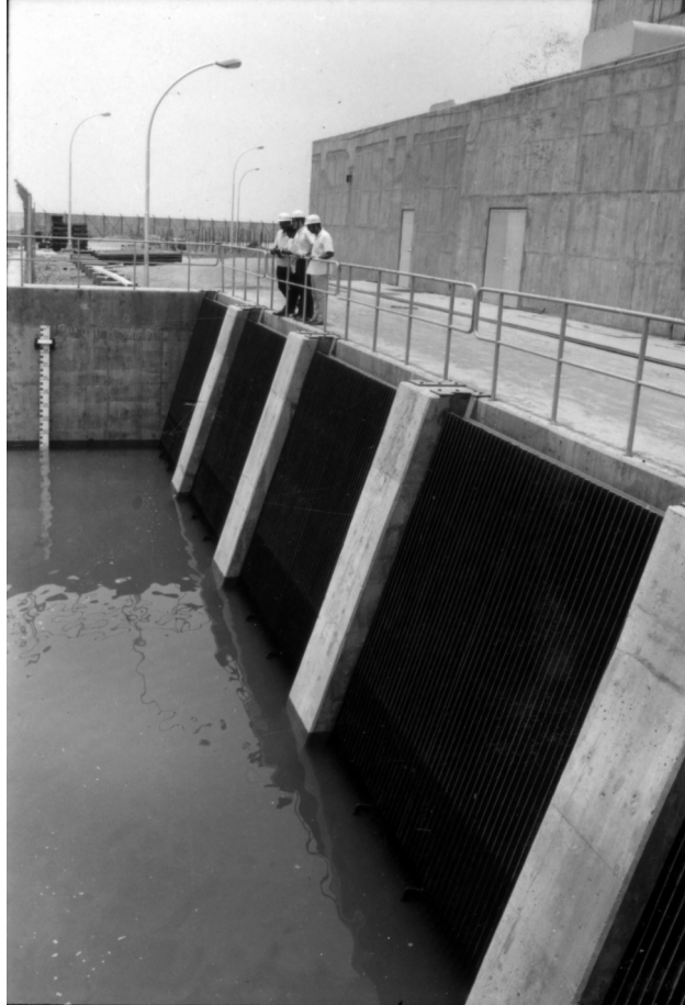
Figure 14. View of the cooling water intake structure on the west side of the plant. (Source: Photographs of Assistance Programs in Foreign Countries, RG 286-CP, NARA.)
