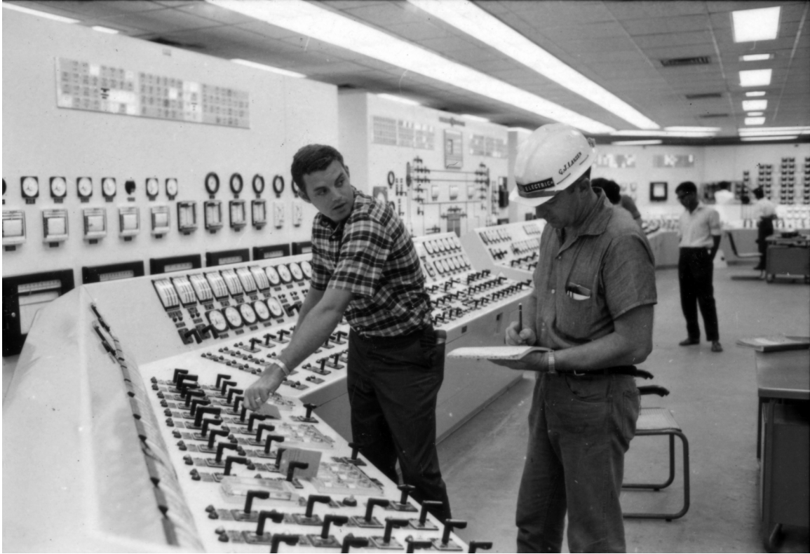
Figure 15. Don T. Spangenberg and G.J. Larsen of General Electric in the Tarapur control room. (Source: Photographs of Assistance Programs in Foreign Countries, RG 286-CP, NARA.)
