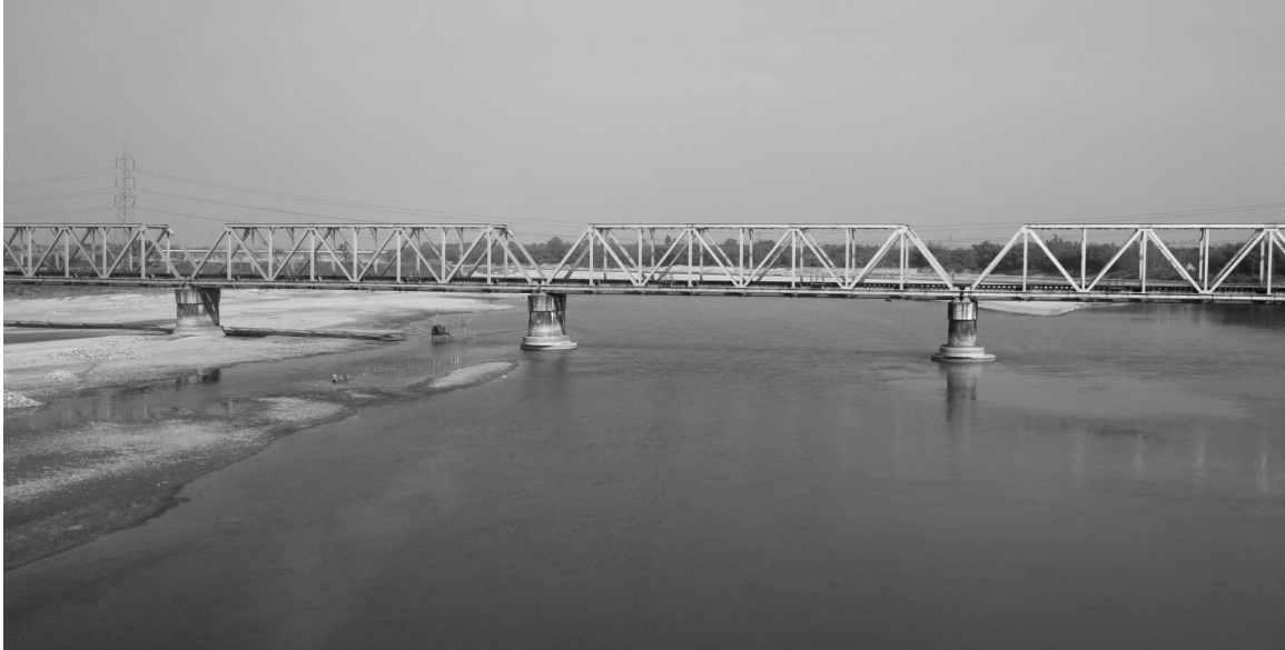
Figure 6. The Sankosh River Bridge on the Assam Rail Link in 2015. The spans are single Warren trusses. (Photo by the author.)
