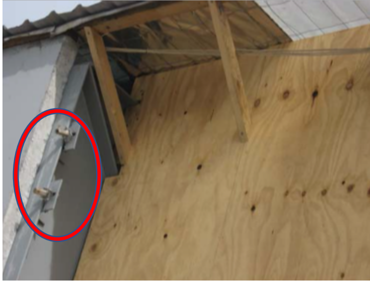
Figure 2-1: Concrete Anchor Connection Failure (Marshall 2012)
