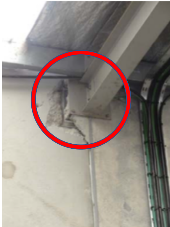
Figure 2-2: Damaged Connection at the Beam-to-Panel Interface (Marshall 2012)
