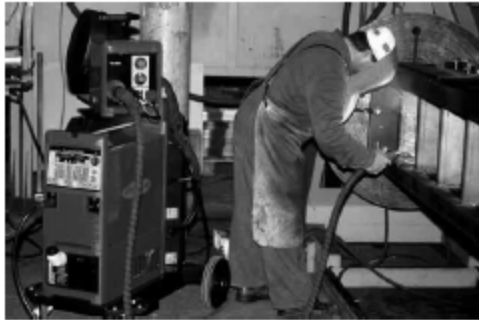
Fig. 20: Digitally controlled 400 A inverter power source being used for steel construction work
