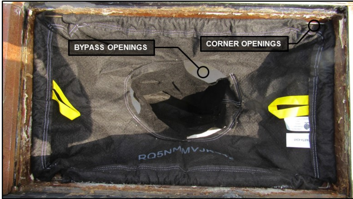
FIGURE 4.15 Openings in Storm Sentinel allow untreated bypass.
