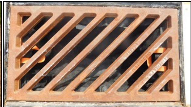
(f) catch basin grate
