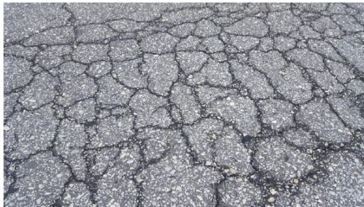
Figure 7. Bottom-Up Fatigue Cracking Example (Vrtis, 2017)
