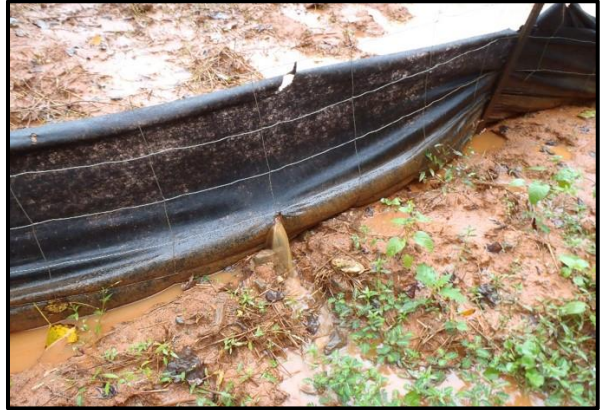
(b) uncontrolled discharge
