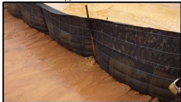
(h) undermining of modification 2
