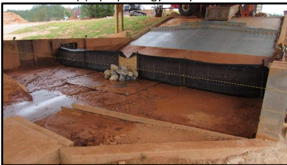
(e) M9 downstream erosion
