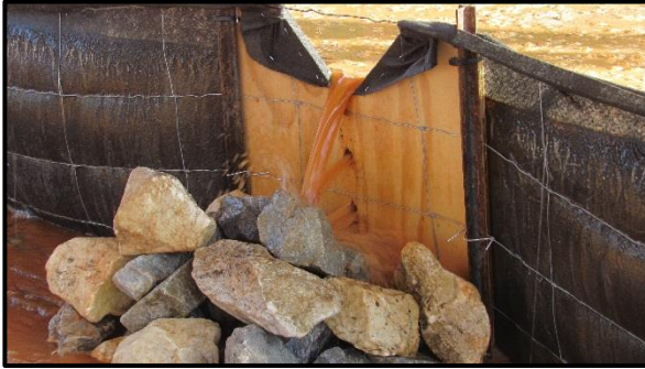
(c) riprap energy dissipater
