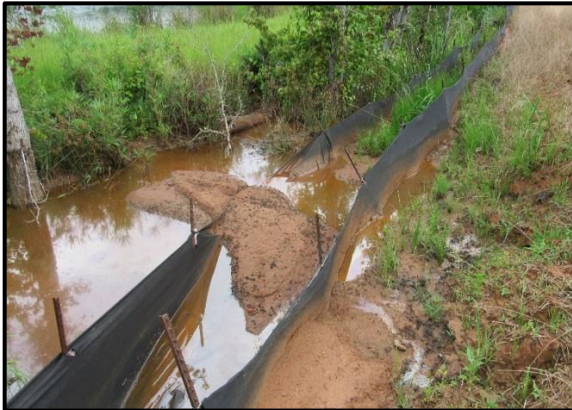
(e) sediment accumulation
