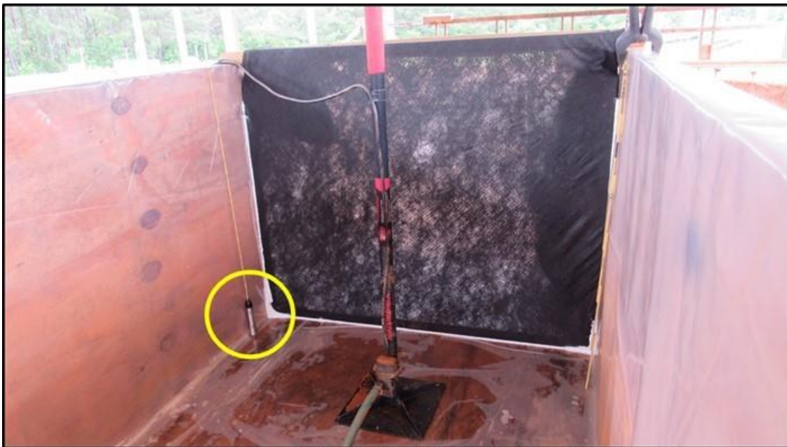
Figure 6.6. Upstream water level logger installation location.
