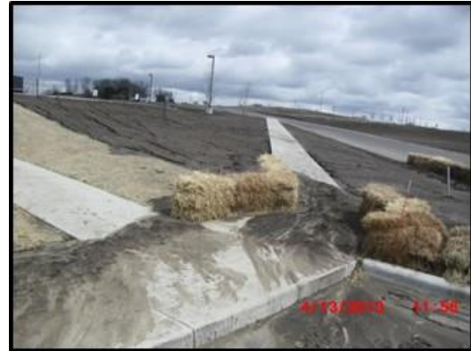
(b) poor installation
