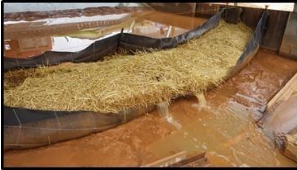
(a) ALDOT SRB overtopping
