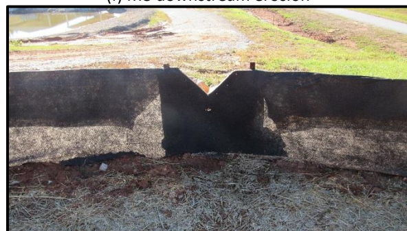
(h) field installation - upstream
