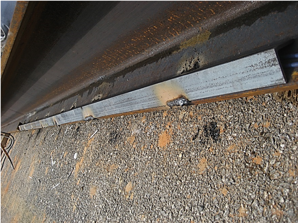
Figure 4-4 – Subsurface Strain Gage Protection
