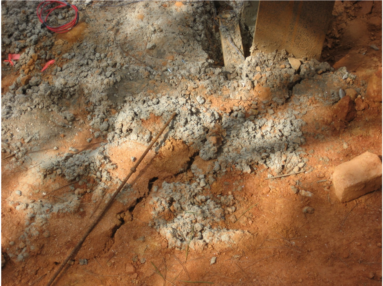
Figure 4-53 – Ground Crack Due to Lateral Load
