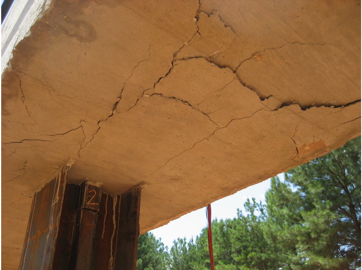
Figure 4-41 – Cracking below the Bent Cap
