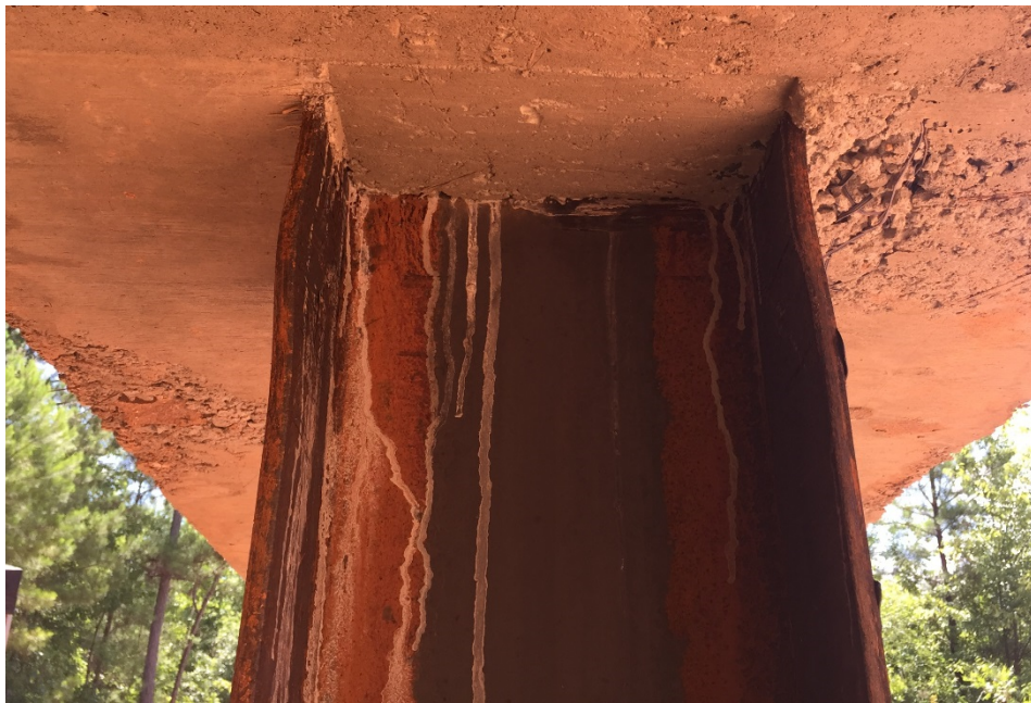
Figure 4-52 – Pile 7 Vertical Flange Buckling
