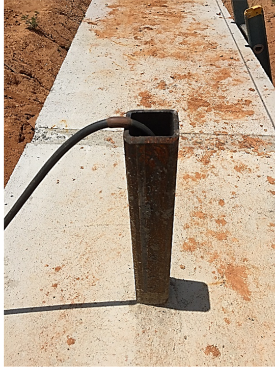
Figure 4-12 – Inclinometer Casing with Inclinometer Downhole
