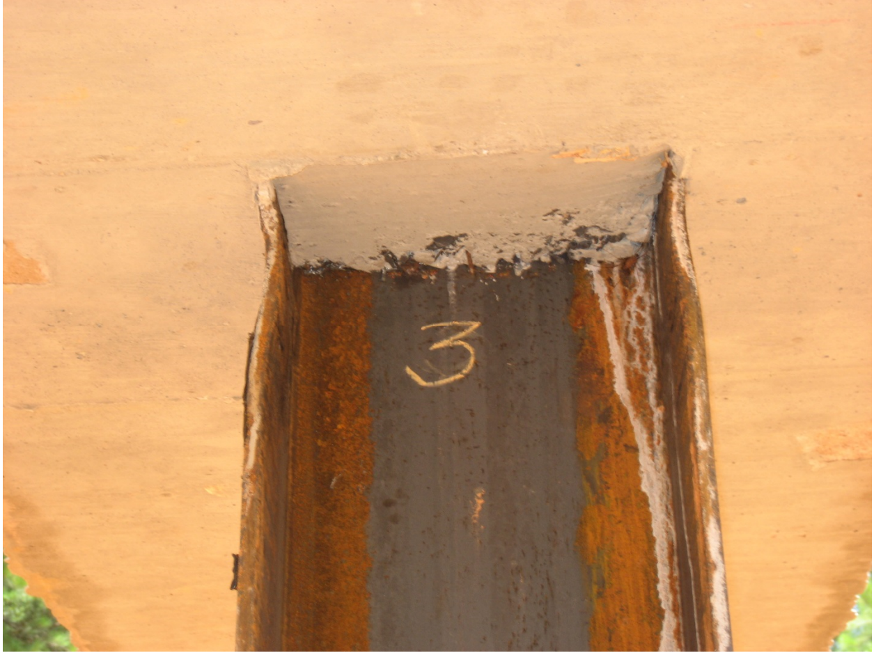
Figure 4-42 – Flange Buckling at Pile 3
