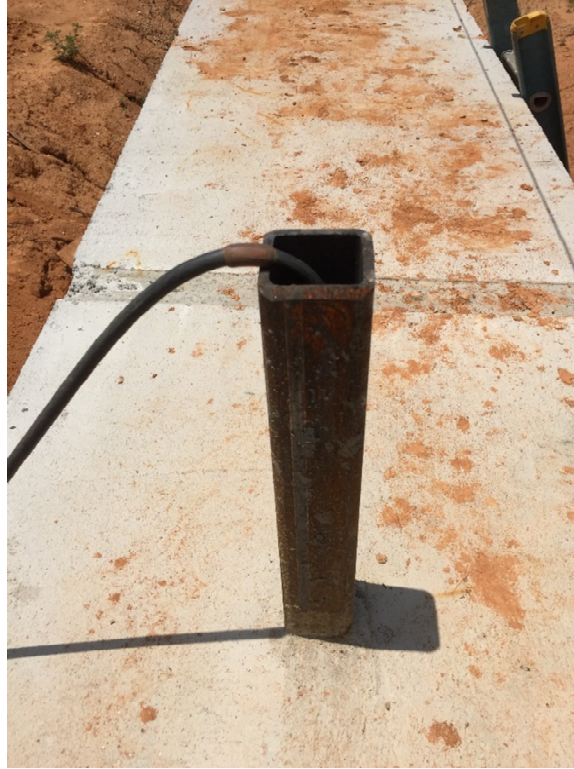
Figure 4-38 – Inclinometer Downhole at Pile 2
