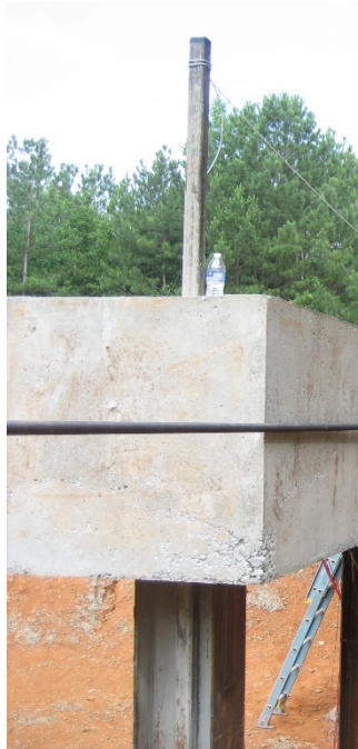
Figure 4-47 – Inclinometer Casing on Pile 5
