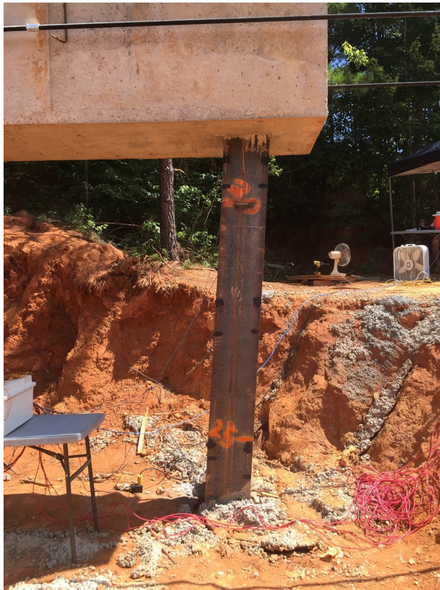
Figure 4-50 – Lateral Deflection Induced in Pile 5 during Field Load Testing
