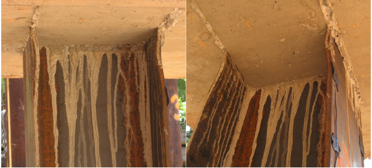
Figure 4-51 – Pile 5 Vertical Flange Buckling
