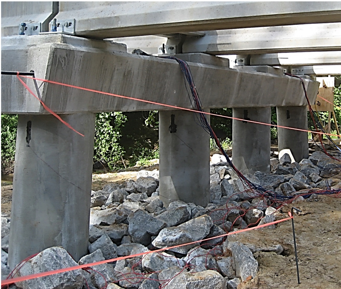
Figure 4-14 – Macon County Road 9 Bridge Test Bent prior to the Casting of the Bridge Deck
