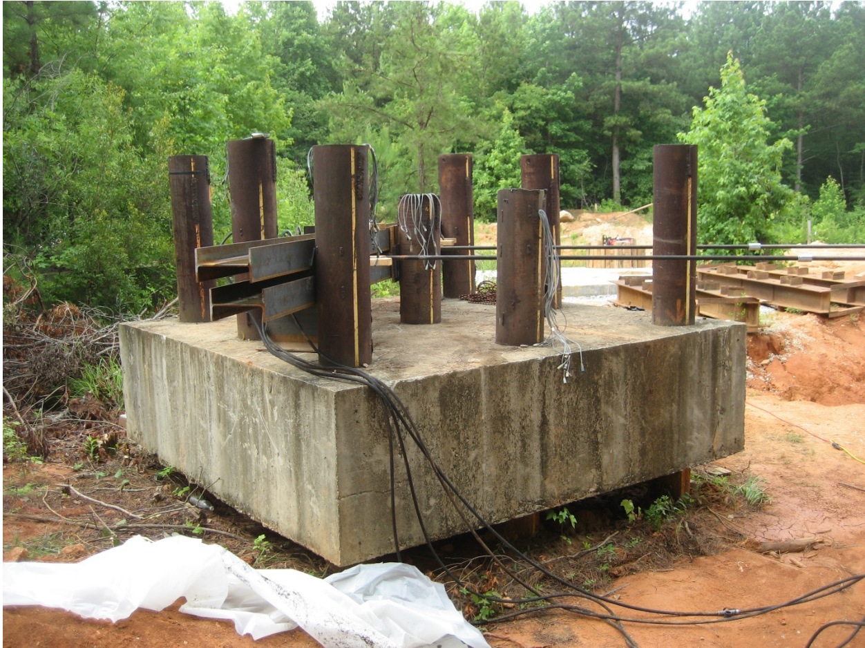
Figure 4-49 – Reaction Pile Group with W10x23 Load Beams (Brown, O'Neill, McVay, El Naggar, & Chakraborty, 2001)
