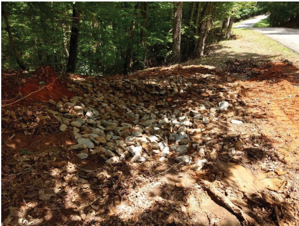
Figure 11: Excavation of outcrops by Public Works Department crew (top) and an example of erosion control measures implemented at the site (bottom).
