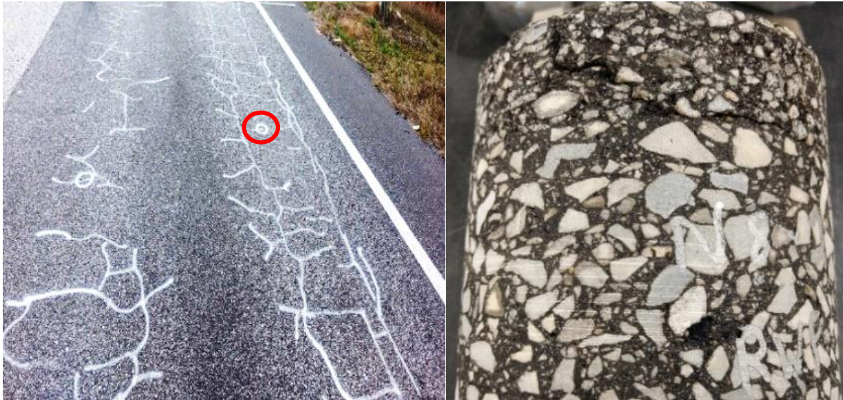
Figure 7. 1 Cracks on Section N8 and Field Core
