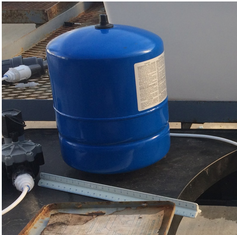
Figure 38: Five Gallon Accumulator Tank Used in HPA Prototype.
