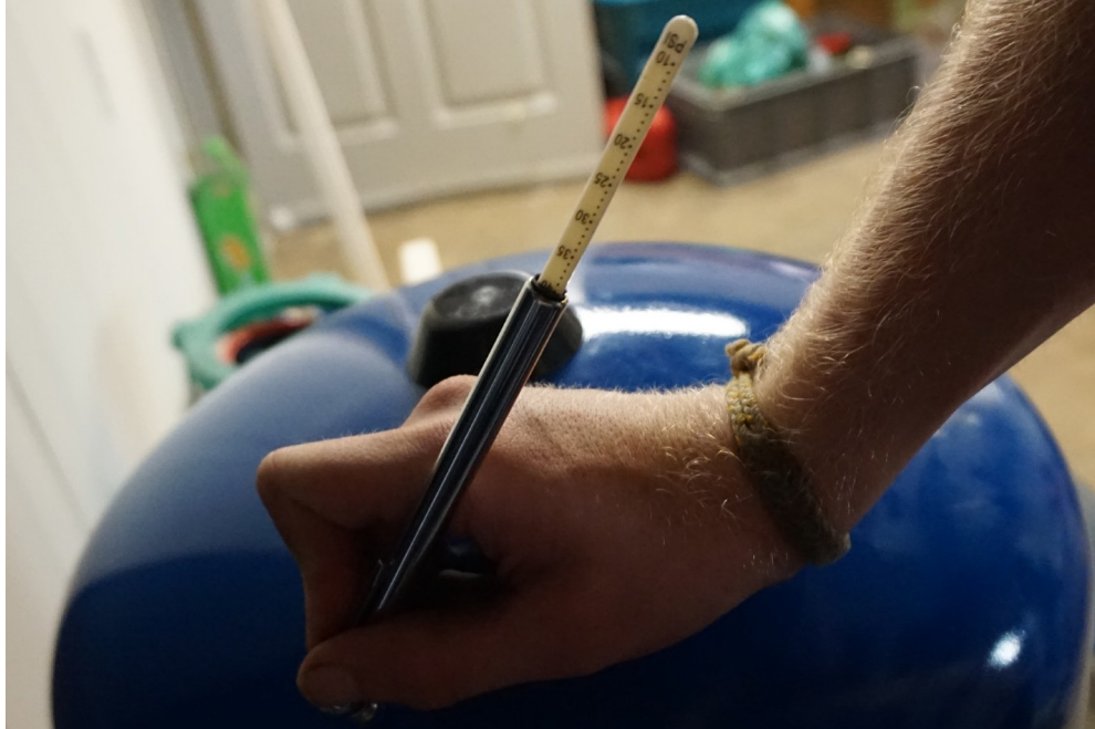
Figure 39: Measuring of Initial Pressure of 26 Gallon WaterWorker Accumulator Tank.
