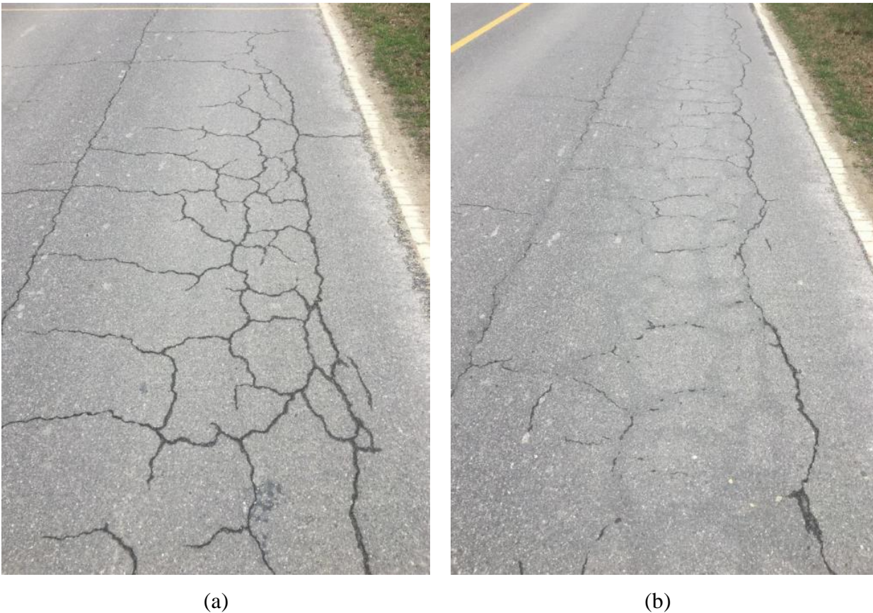
Figure 4-4 cracking in (a) micro surfacing and (b) micro surfacing with crack sealing in advance (133)
