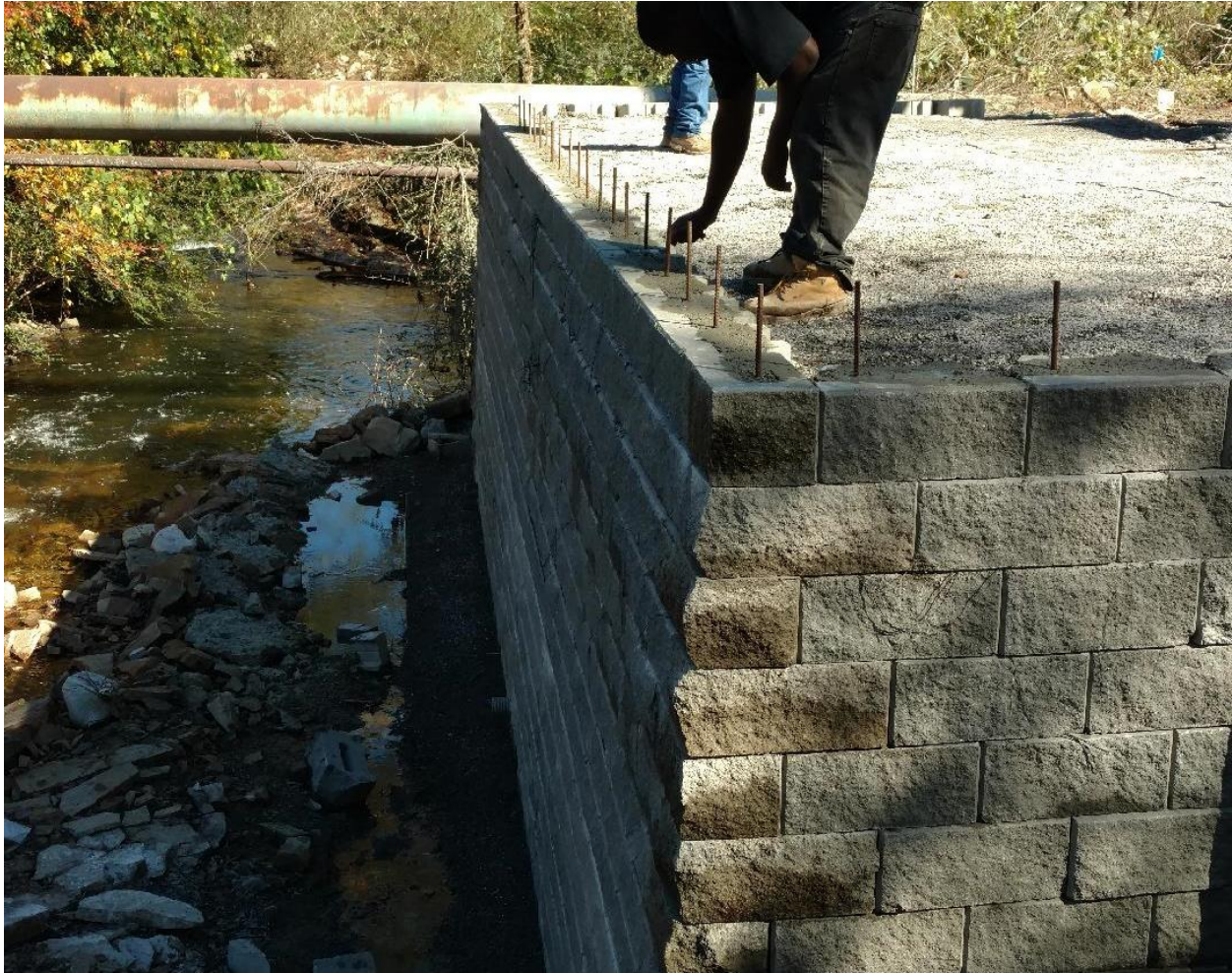
Figure 35. 16 th course of east abutment. This is the second of the top three rows, which were pinned with No. 4 rebar and grouted with ready-mix cement.
