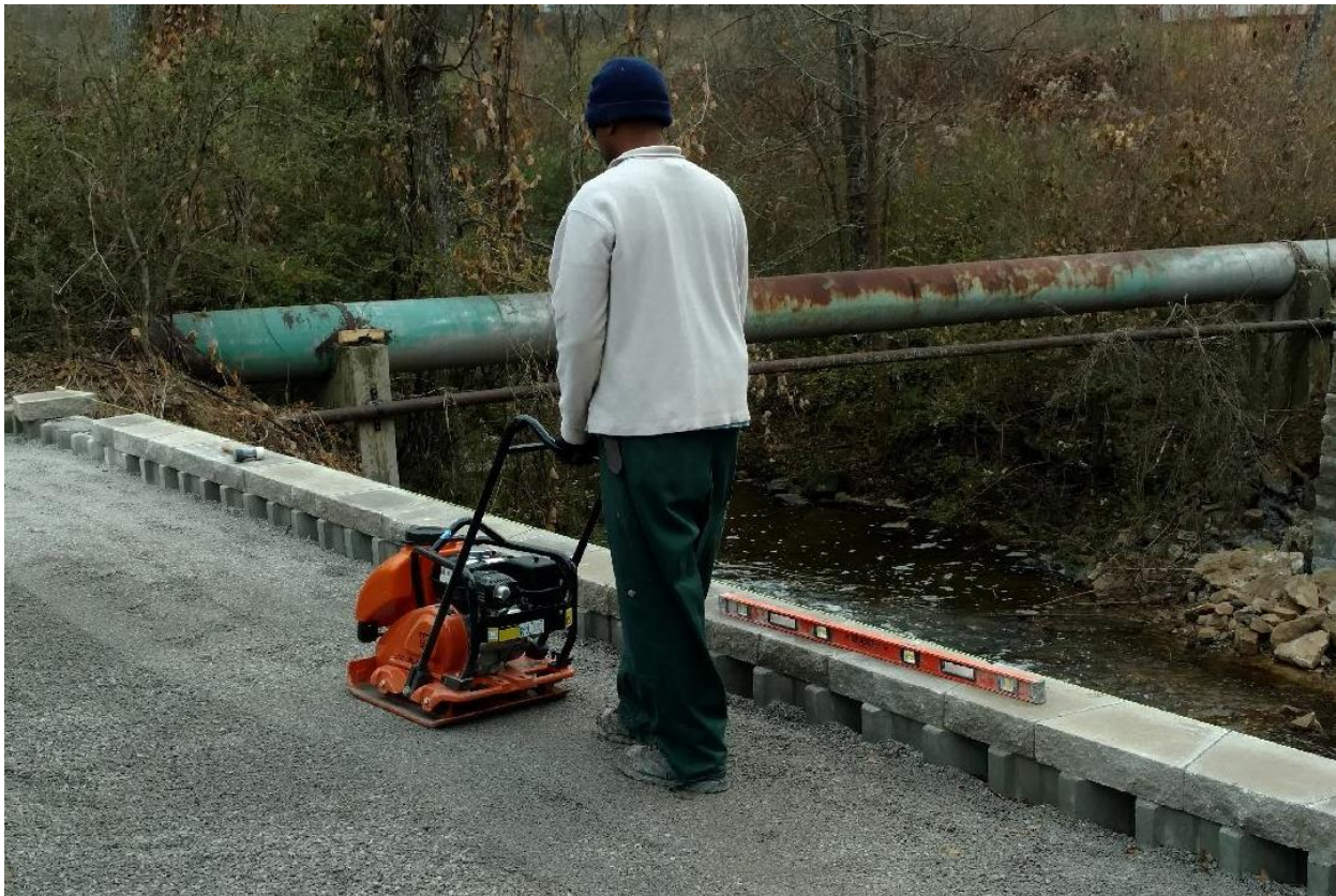
Figure 17. Worker using a walk-behind vibratory plate tamper to compact backfill while constructing the Turkey Creek GRS-IBS in Marshall County, AL.
