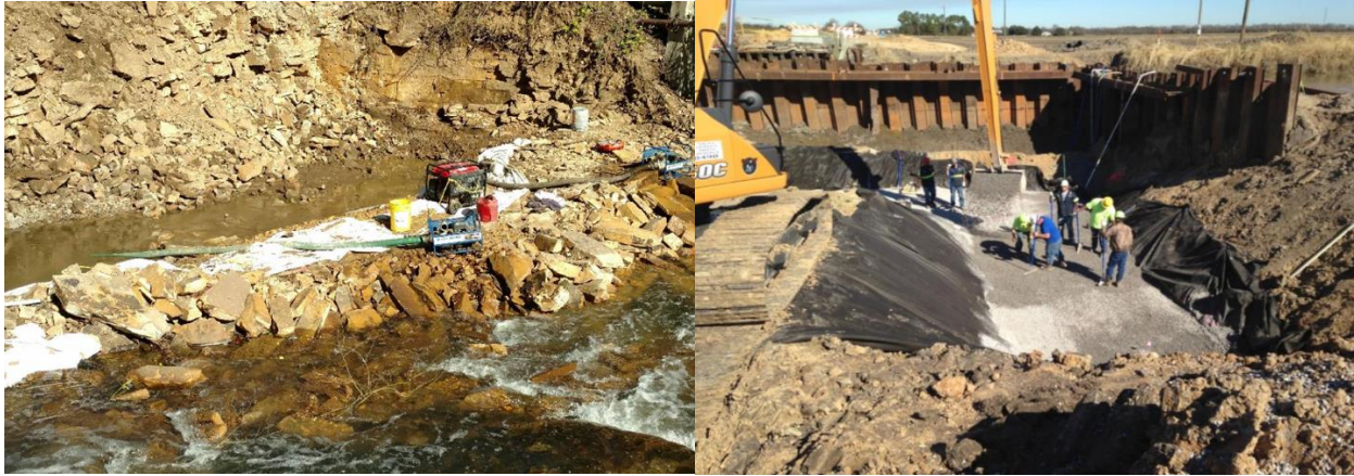
Figure 18. (a) Dewatering pumps used to remove flooded excavation at Turkey Creek bridge in Marshall County, AL; (b) reinforced soil foundation constructed inside a cofferdam at Maree-Michel bridge in Vermilion Parrish, LA.
