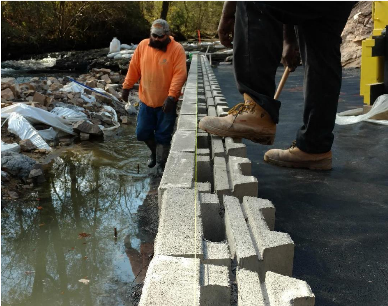
Figure 19. A string line being used to check the line and grade of the 6 th course of the west abutment.
