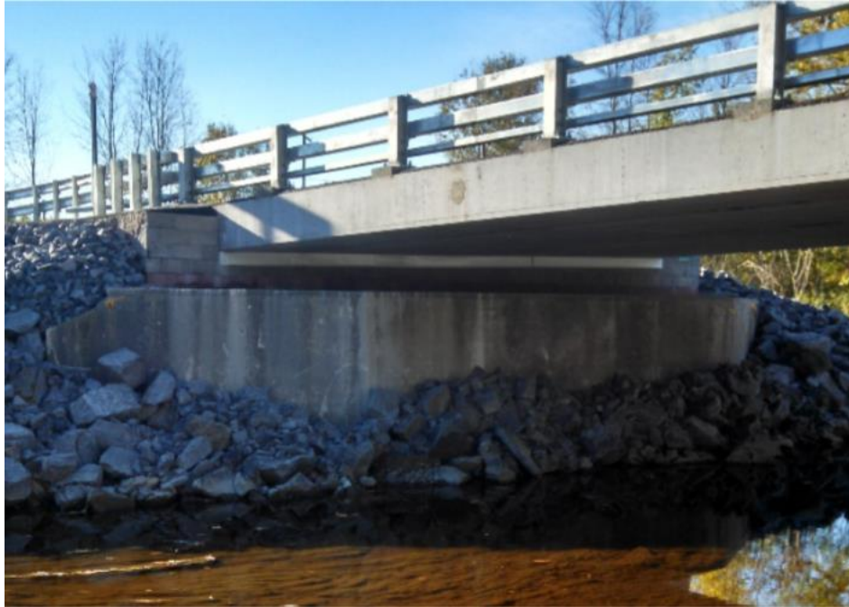
Figure 15. Elliot Road GRS-IBS in St. Lawrence County, New York State. A setback GRS “stub wall” was built atop the existing (south) concrete abutment.
