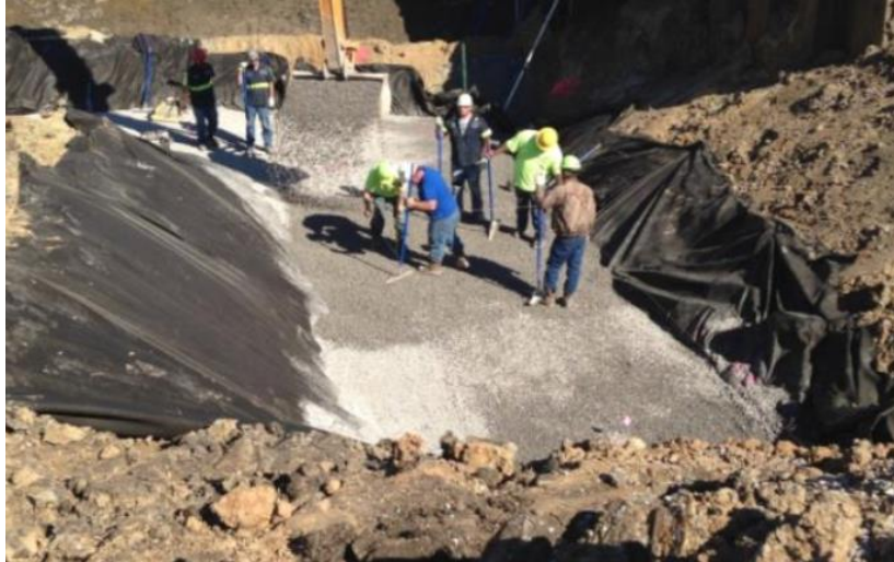
Figure 4. Construction of a reinforced soil foundation for the Maree-Michel bridge in Vermilion Parish (LaDOTD 2016)
