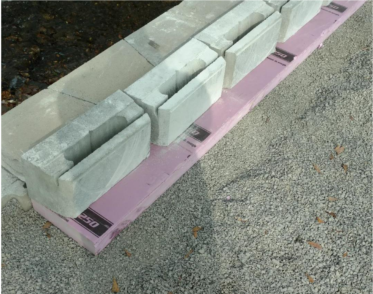
Figure 37. Polystyrene foam board used to provide 3 in. of clear space for the east abutment beam seat.
