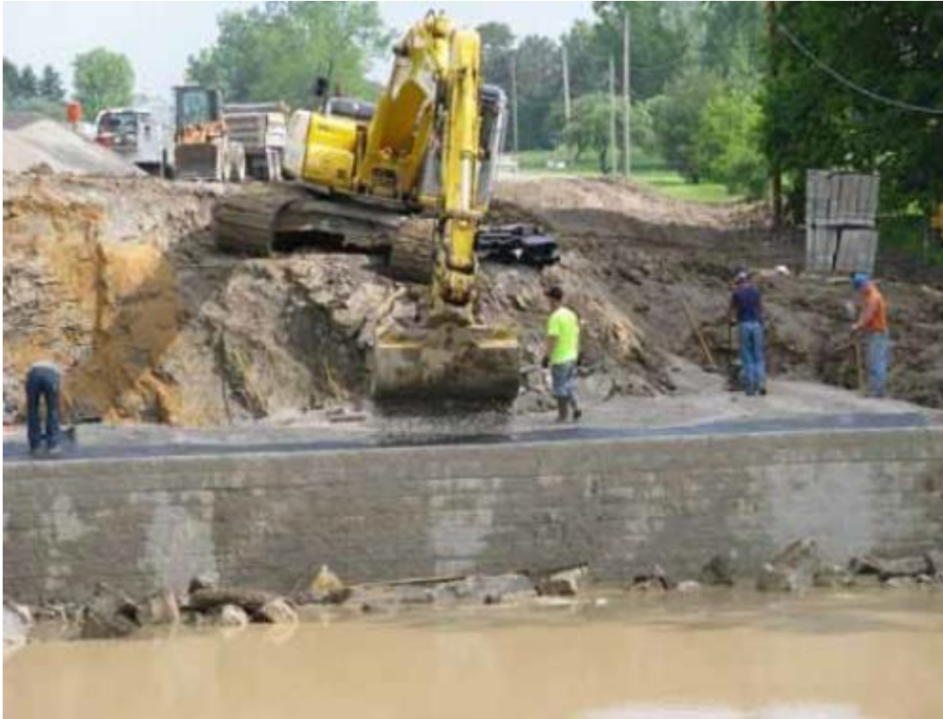
Figure 3. GRS-IBS abutment under construction in Defiance County, Ohio (Adams et al. 2011a)
