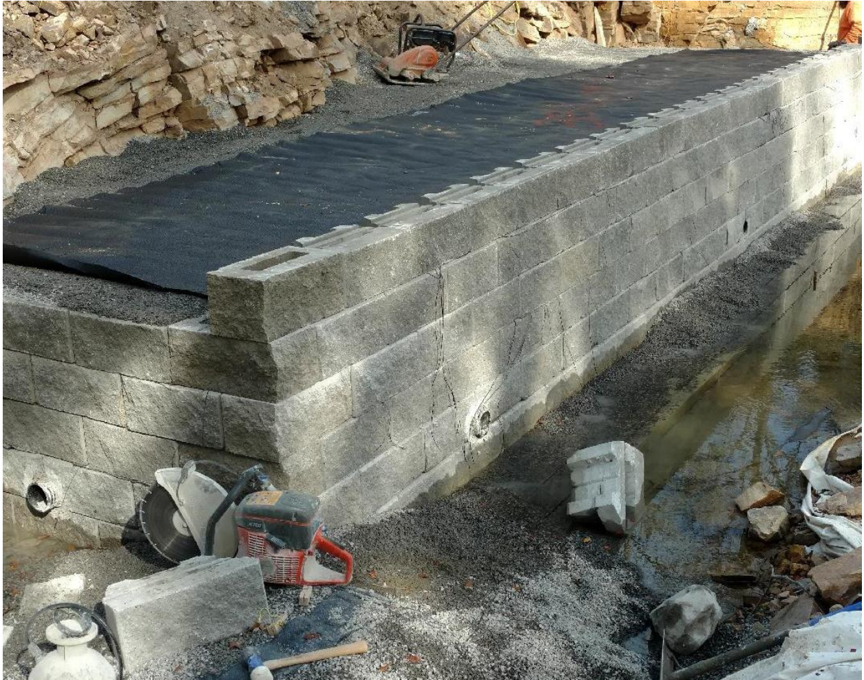
Figure 34. 6 th course of west abutment. Masonry SRW block joints were offset between courses to minimize seams within the wall face.
