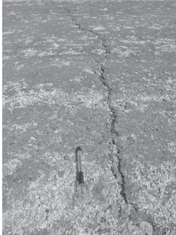
Figure 2.2 Cement Treated Pavement Section with Shrinkage Cracks (Sebesta, 2005).
