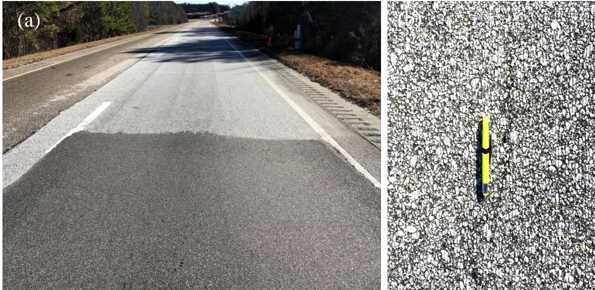
Figure 5.6 The Surface of Section S9. (a) Pavement Section Surface View, (b) Visible Cracks at S9 (Date Taken: 02/07/2021).
