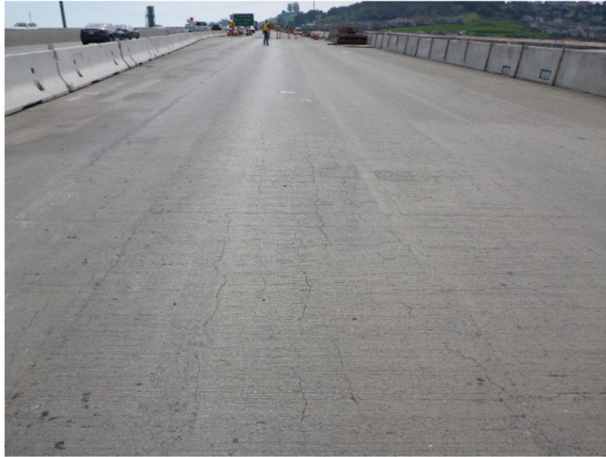
Figure 1-3. Longitudinal deck cracks (Caltrans)
