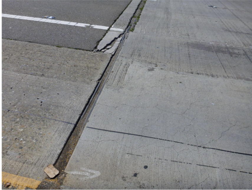
Figure 1-4. Map pattern cracks (Caltrans).
