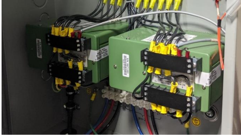
Figure 3.22: AC watt transducers
