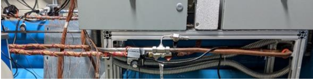
Figure 3.17: Electric preheater section
