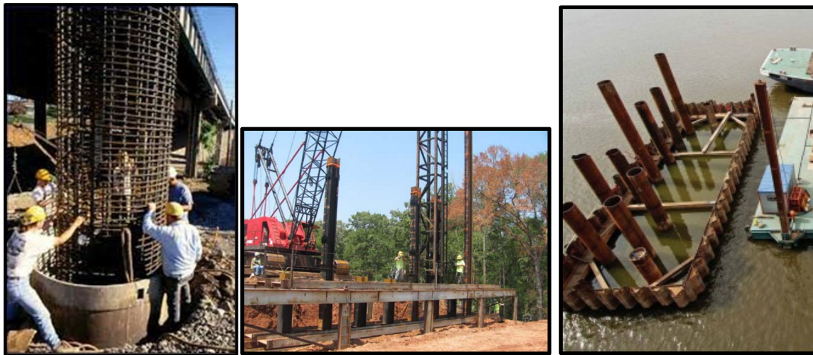
Figure 1.1. (a) RC drilled shaft Steel [1]; (b) HP piles [2]; (c) Large diameter steel piles [3]
