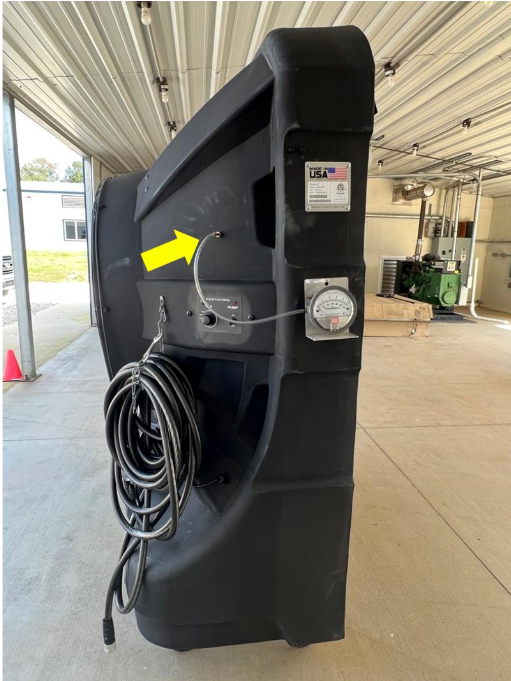
Figure 2: Pressure across the pads was taken with a differential pressure gauge mounted to the side of the unit. The yellow arrow indicates the negative pressure port location.
