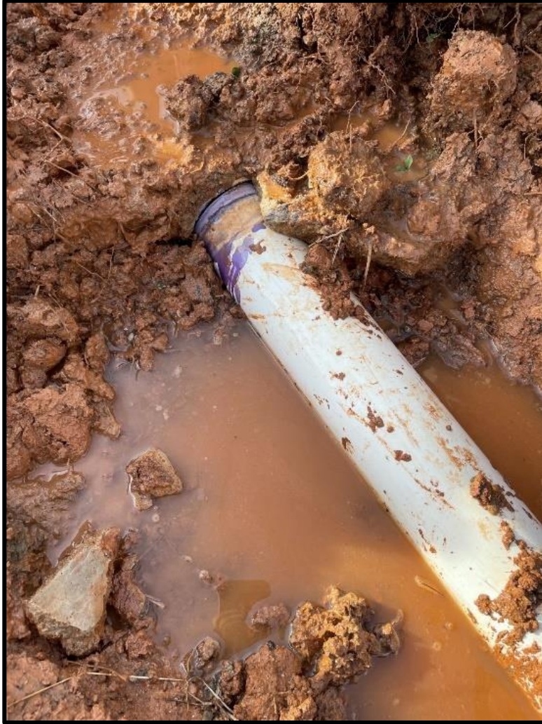
Figure 3-19: Failed PVC Connection
