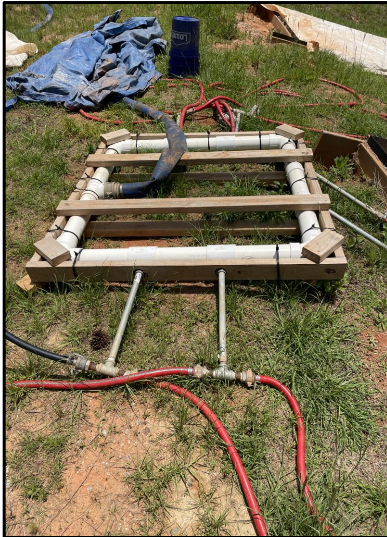
Figure 3-13: Original Water Supply Manifold
