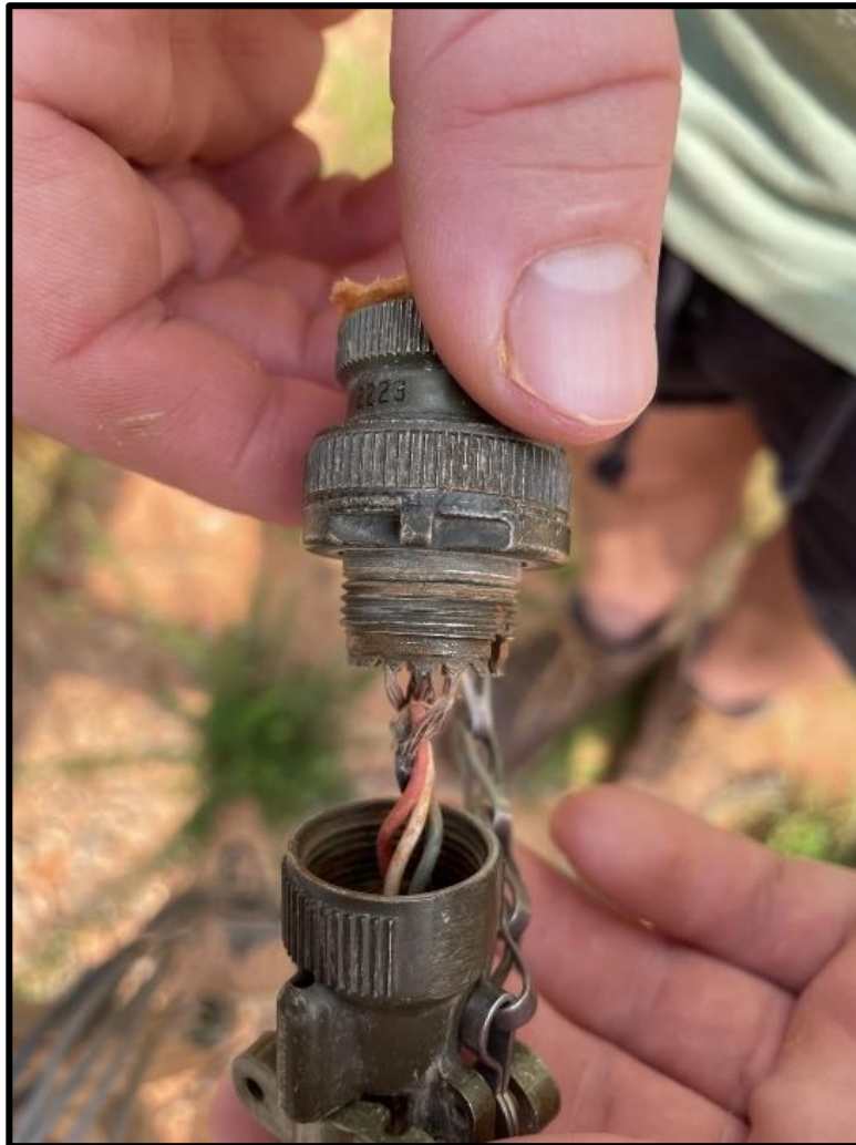
Figure 3-15: Solenoid Valve Wiring Without Insulation
