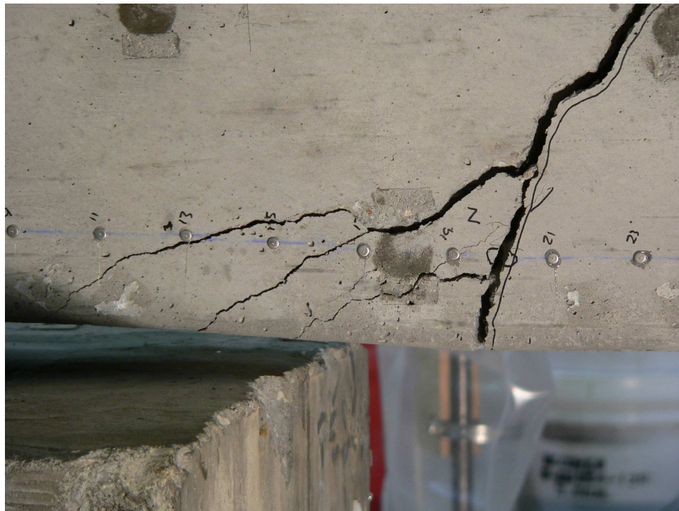
Figure 4-4. Shear tension failure showing loss of bond - STD-M-E
