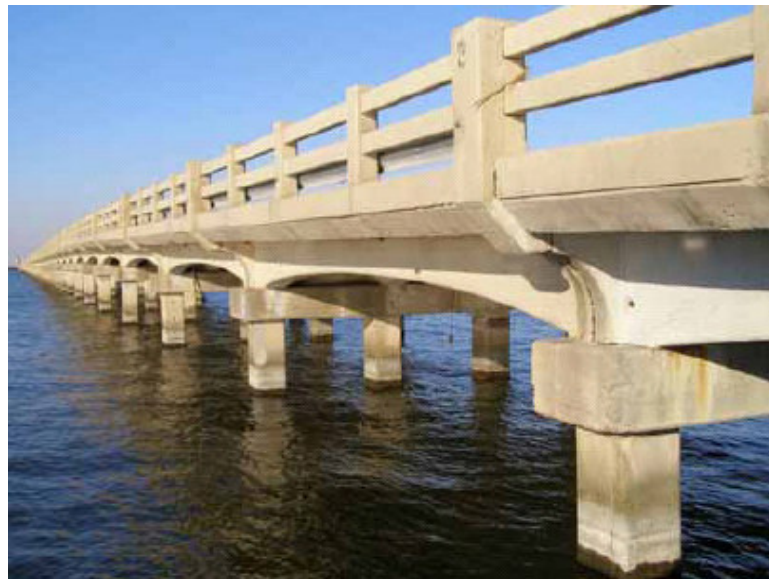
Figure 2.4 Cast-in-place concrete bridge carries the traffic of US-11 over Lake Pontchartrain (photo credit: J. O'Connor, MCEER) (NIST, 2006).
