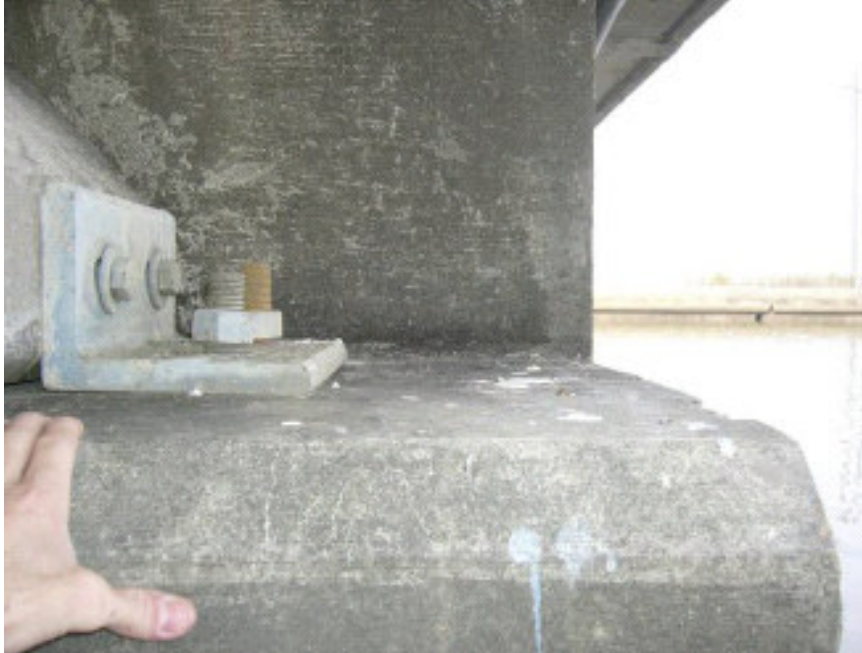
Fig. 2.32 Photo of clip angle connection that did not fail on another part of I-10 on-ramp near Mobile (Douglas et al, 2006).
