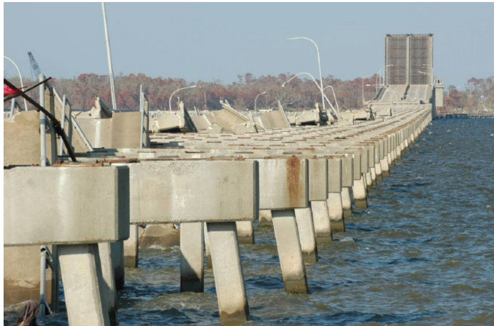
Fig. 4.12. Photograph of the damage to the U.S. 90 Biloxi Bay bridge caused by Hurricane Katrina. Photo was taken looking northeast from Biloxi 9/21/05 (Katrina Hit 8/29/05).
