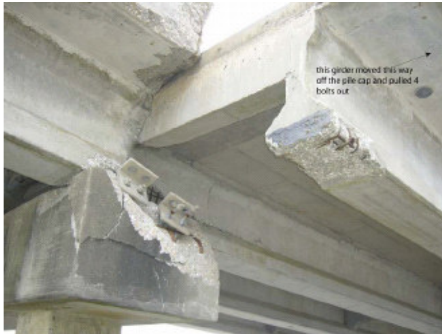
Fig. 2.30 Photo of northeast corner of span #11 of I-10 on-ramp near Mobile, AL (Douglass et al, 2006).
