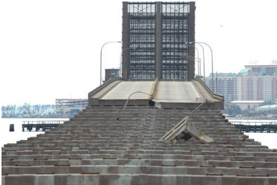
Fig. 4.14. Photograph of U.S. 90 bridge over Biloxi Bay showing the westbound half-span #100 that is still on pile caps but rotated and displaced to the landward side. The eastbound half-span was knocked completely off. The spans at higher elevations, beginning with span #99, were not knocked off the pile caps by the storm. (This photo was taken 2/19/06 looking southwest from Ocean Springs towards Biloxi.)
