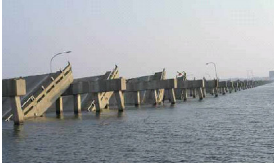
Fig. 3.39 Looking west toward Biloxi from the east shore, many superstructure spans of US-90 Biloxi-Ocean Springs bridge were displaced north off their piers (photo credit: J. O'Connor, MCEER) (NIST, 2006).
