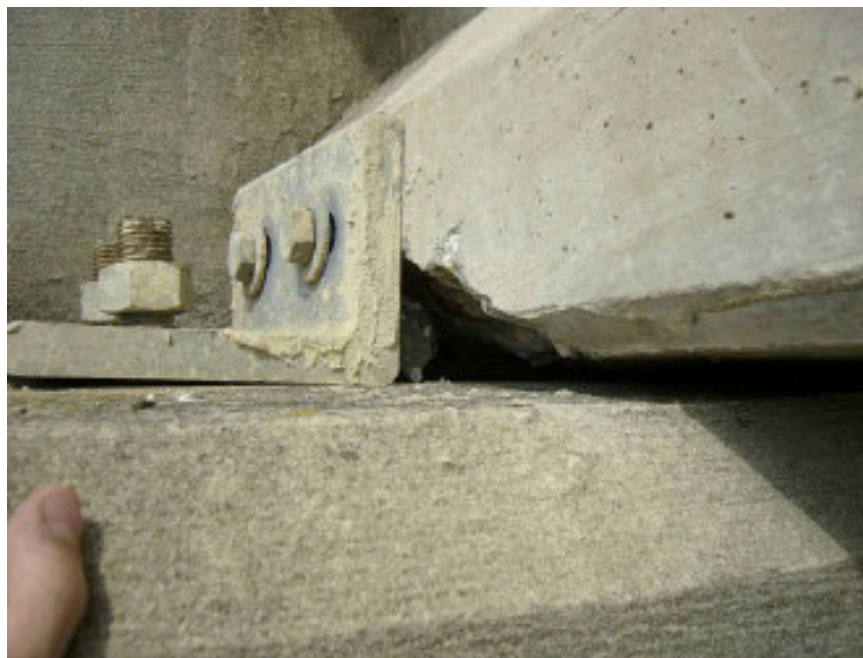
Fig. 2.31 Photo of typical slip angle connection of I-10 on-ramp near Mobile showing failure of concrete around bolts but without subsequent span displacement (Douglass et al, 2006).
