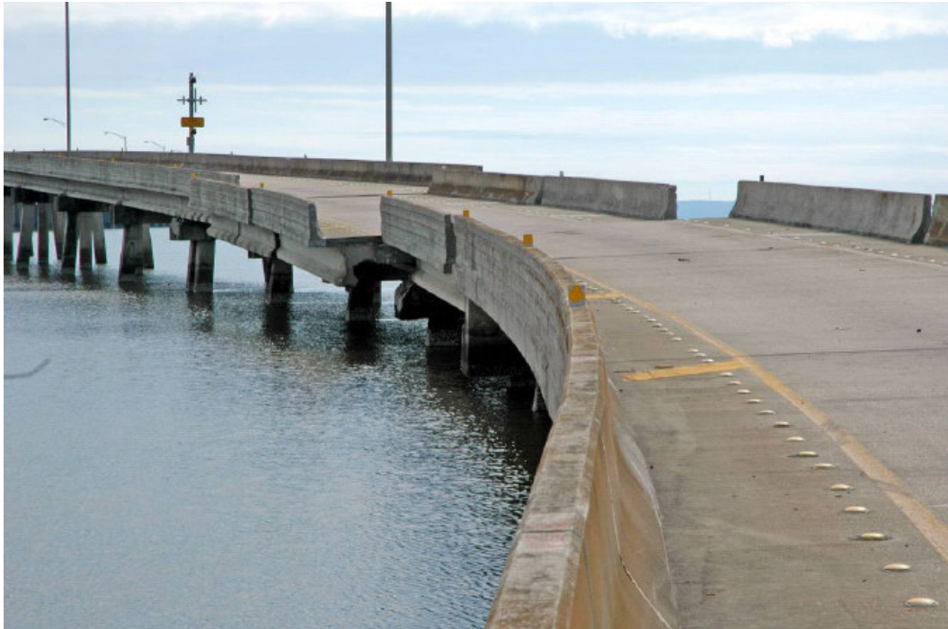
Fig. 2.29 Damage to I-10 on-ramp near Mobile, Alabama, caused by Hurricane Katrina (Douglass et al, 2006).
