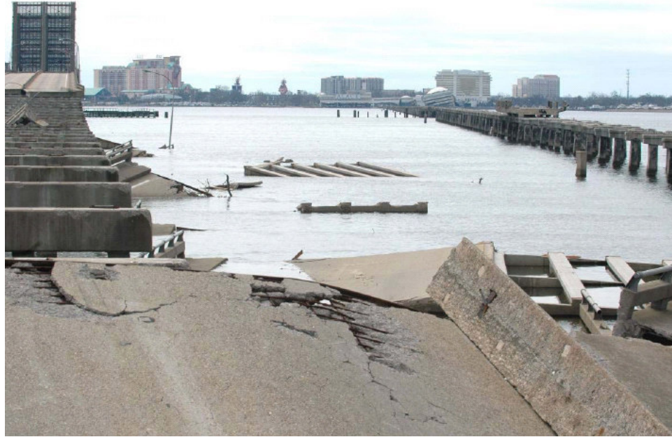
Fig. 4.11. Photo looking west toward Biloxi of Hurricane Katrina damage to U.S. 90 Bridge over Biloxi Bay (from Douglass et al., 2006).
