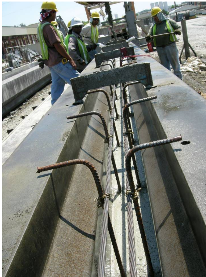
Figure 3-15: SCC Flow from East-End Discharge Point
