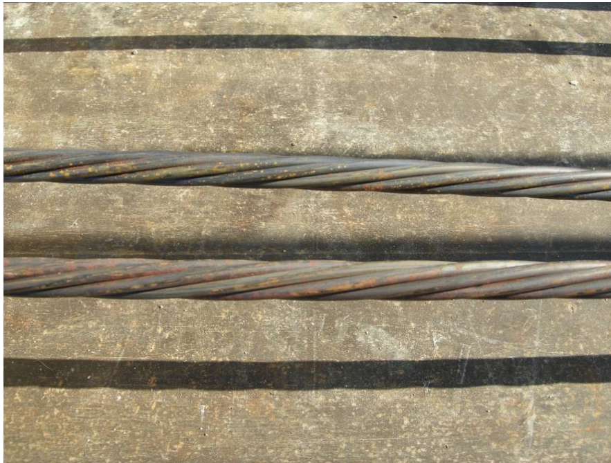
Figure 3-8: Typical Strand Surface Condition
